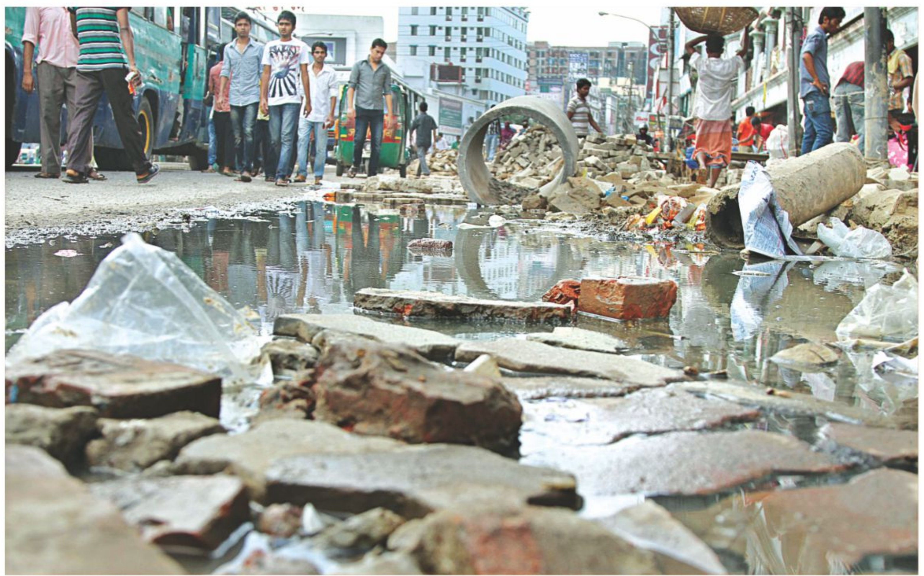
Bits and pieces of pavement and sewerage pipes are left scattered at Farmgate in the capital after authorities dug trenches to carry out repair work. Pedestrians now have to share the street with buses. The photo was shot yesterday. PHOTO: SK ENAMUL HAQ
