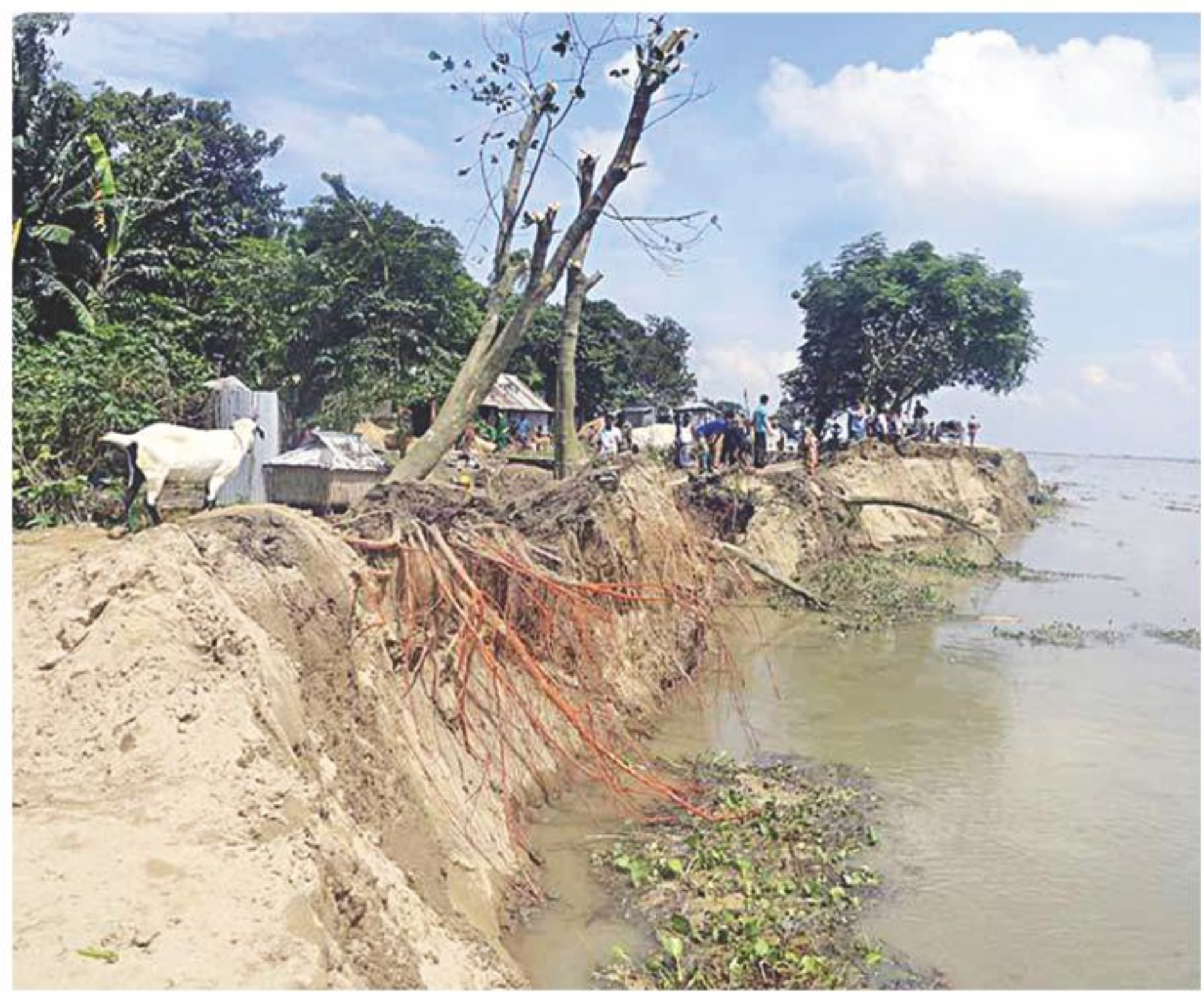
PHOTO: STAR Over 150-metre area of Fulchhari Flood Control Embankment collapsed at Hazarhat in Fulchhari upazila under Gaibandha district yesterday, triggering erosion in the area.
