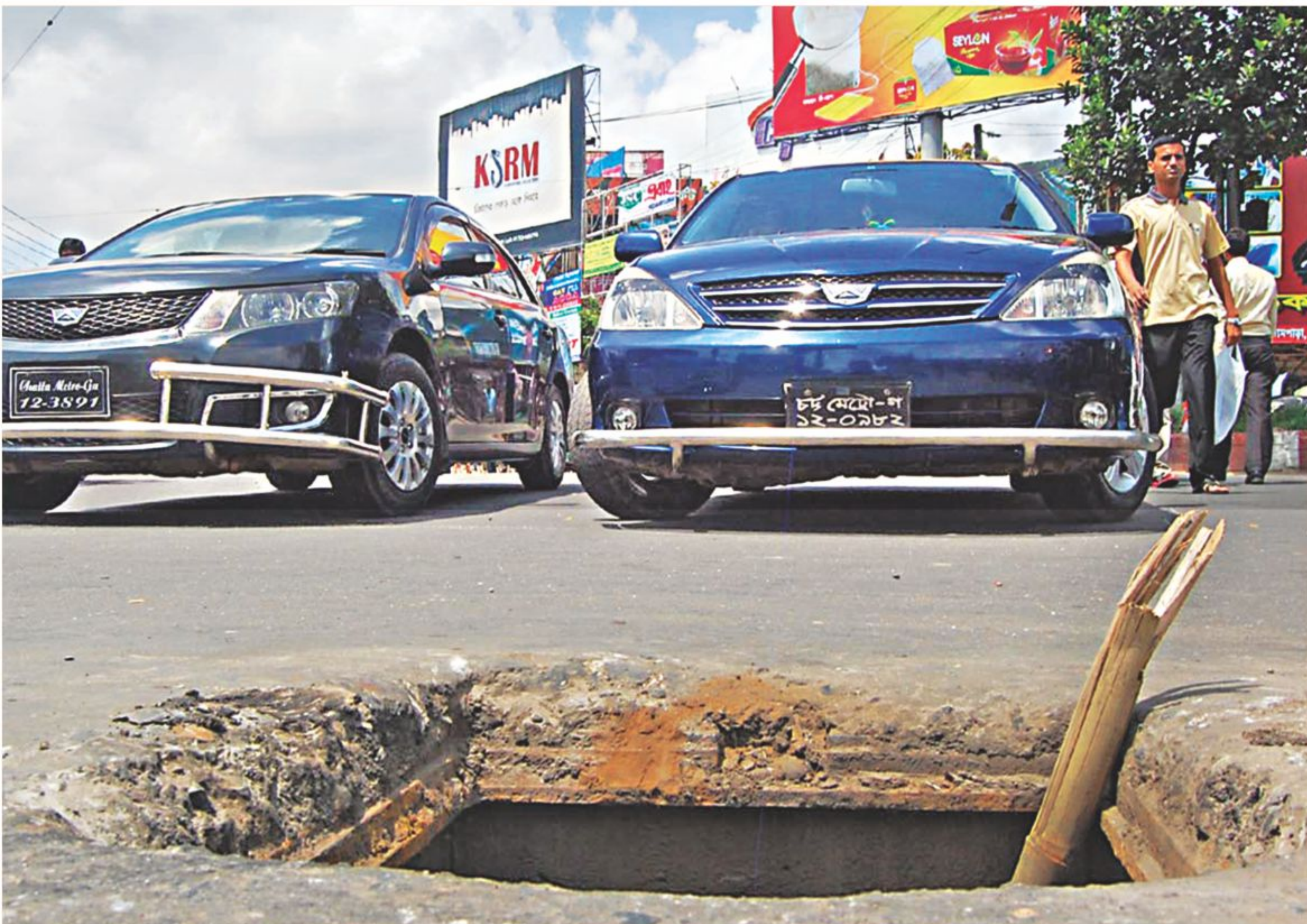
The manhole has been without a lid for about a week at Sholoshahar No 2 Gate intersection in Chittagong city. Pedestrians and vehicles often fall into the manhole at night. Yet the authorities seem blind to the situation.
