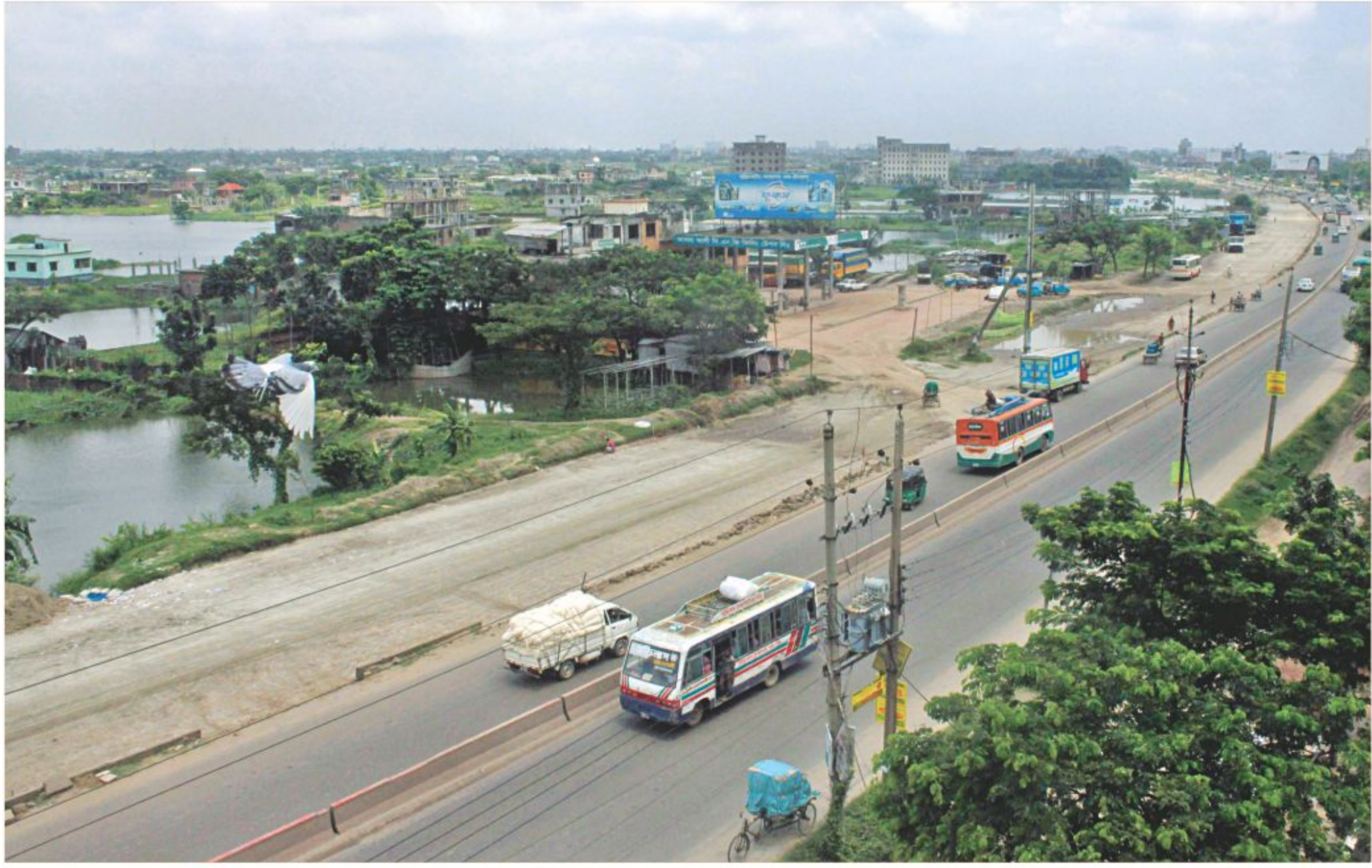
The deadline for widening the Jatrabari-Kanchpur stretch of Dhaka Chittagong highway is June next year but there is little sign that the work will be finished on time. The photo was taken recently.
