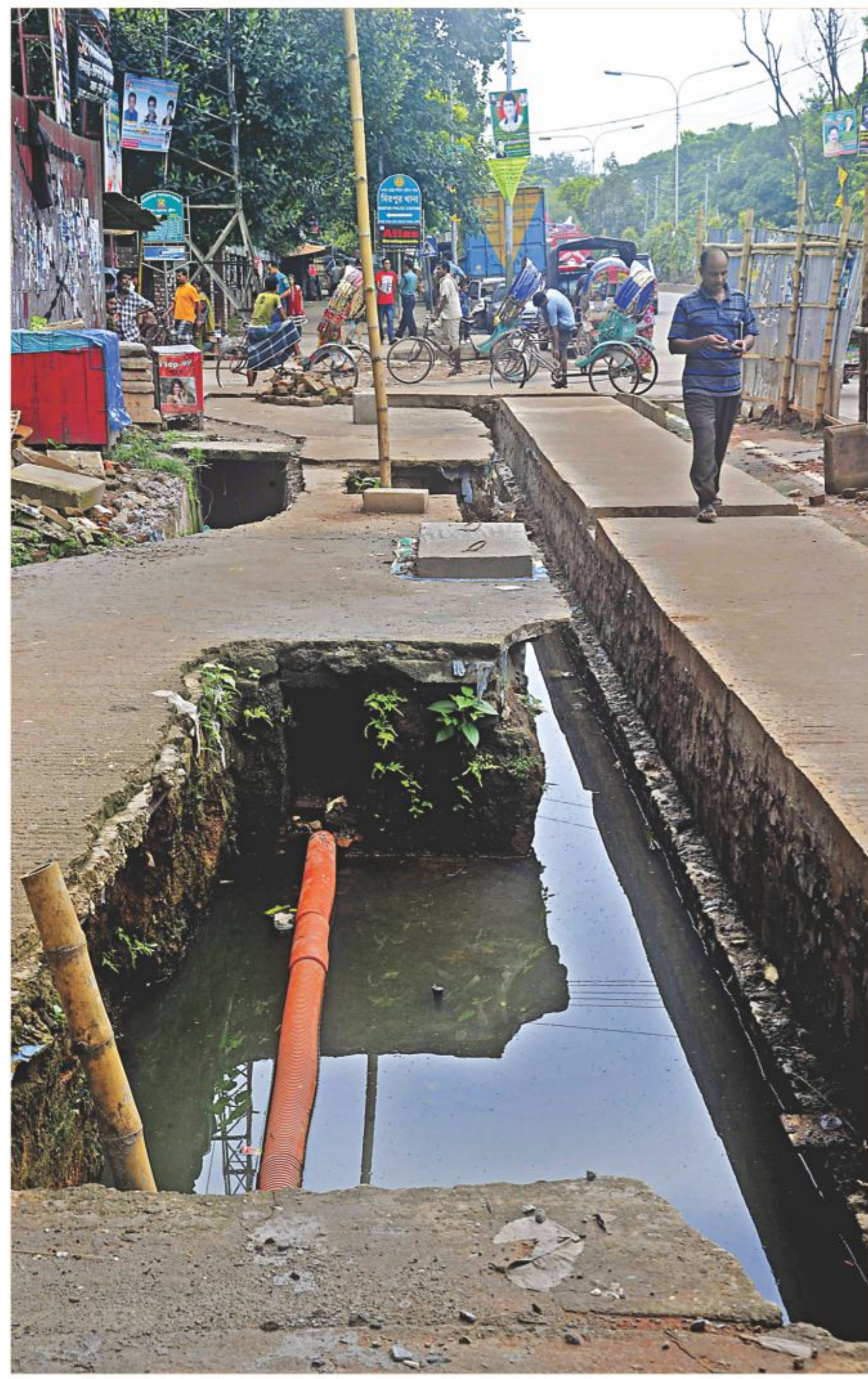
A broken footpath, repair work of which was suspended on the occasion of Eid, still remains unrepaired after the holidays, posing danger to pedestrians. The photo was taken near Mirpur Police Station in the capital yesterday.
