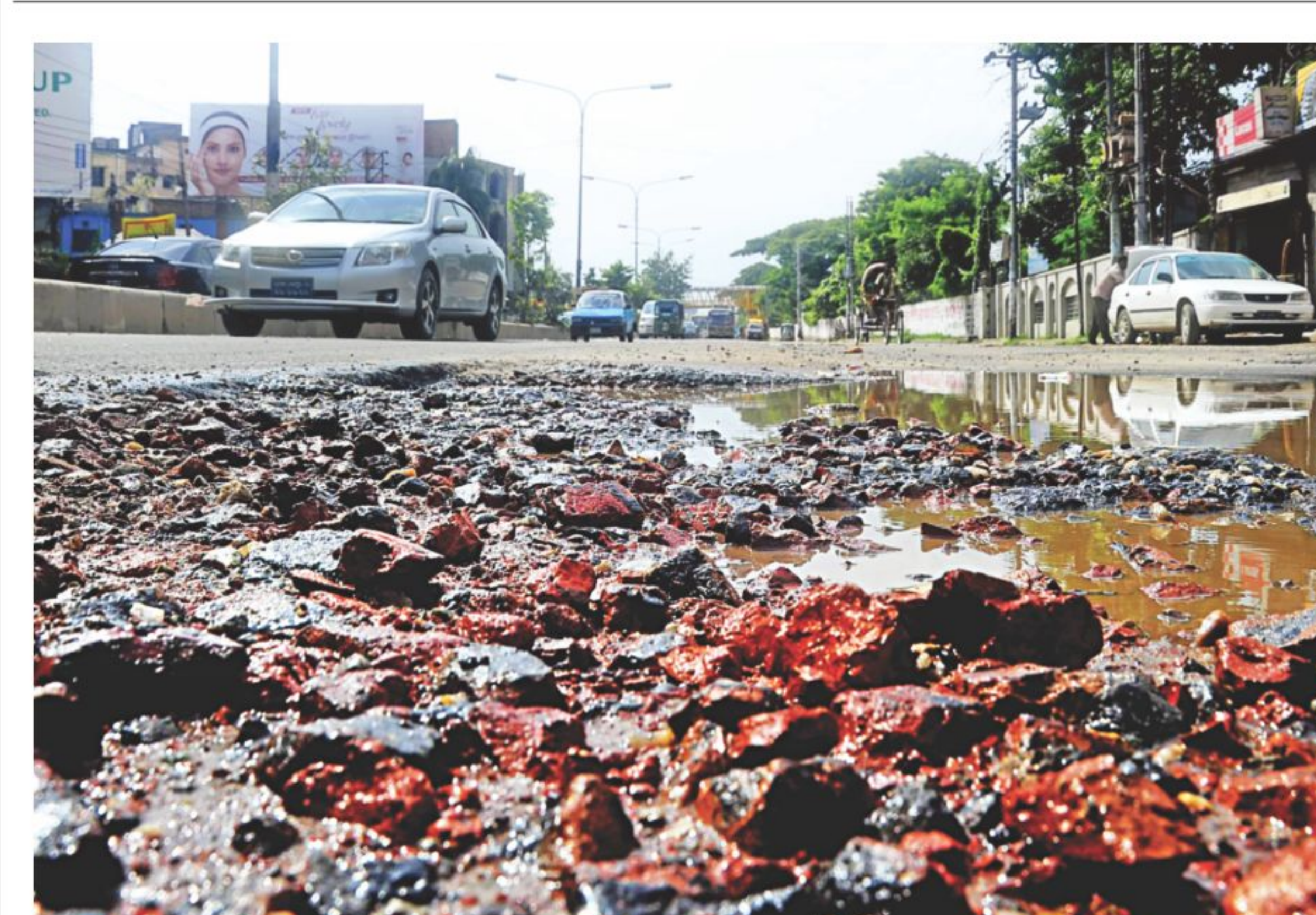
Shabby repair work after Wasa installed a pipe has left Darussalam Road in the capital's Mirpur in a sorry state. The photo was taken on Friday.
