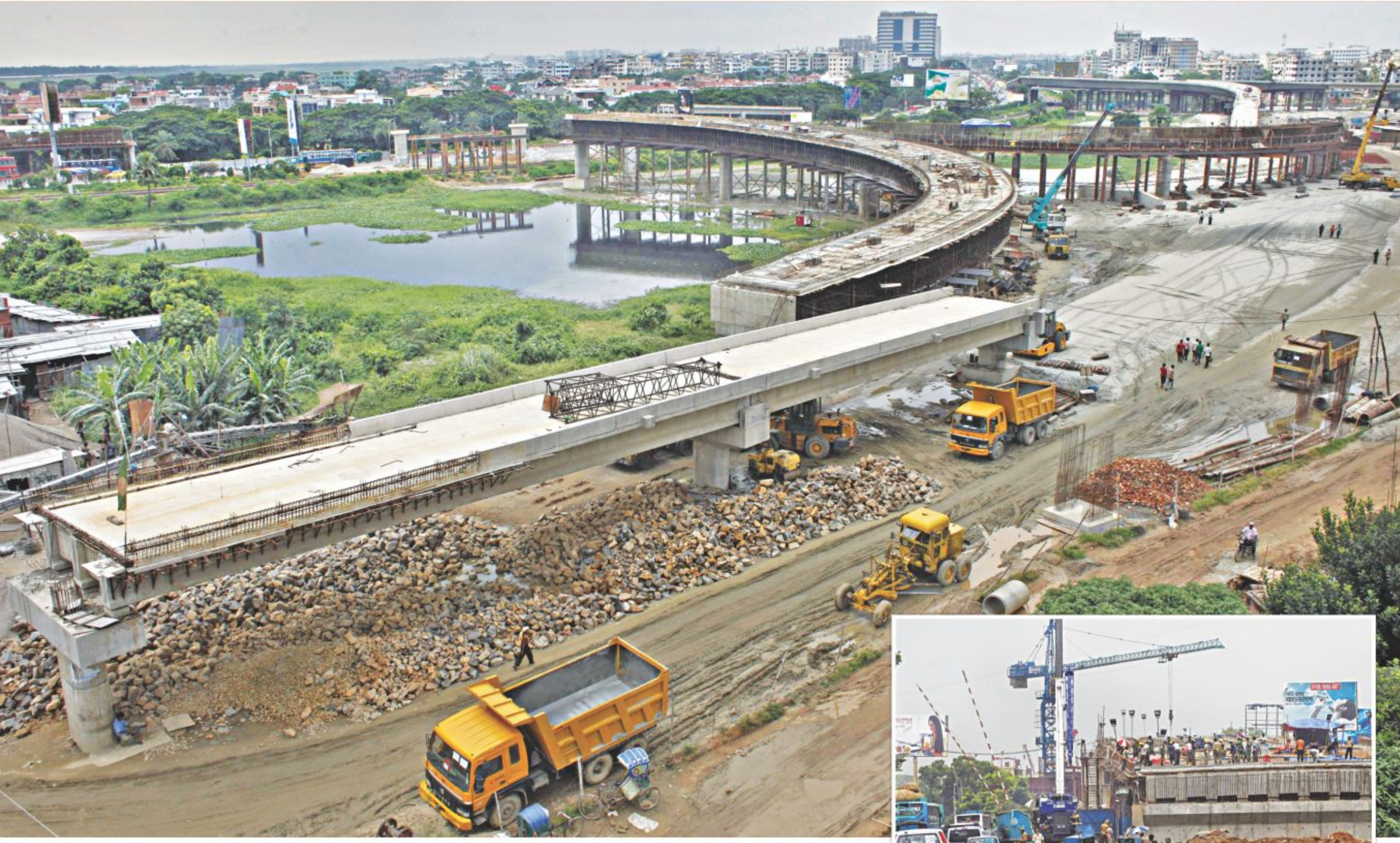
The under-construction Kuril flyover evolving to completion. It is expected to significantly ease traffic congestion in the capital. Inset, workers busy installing a part. The photos were taken yesterday. PHOTO: RASHED SHUMON
