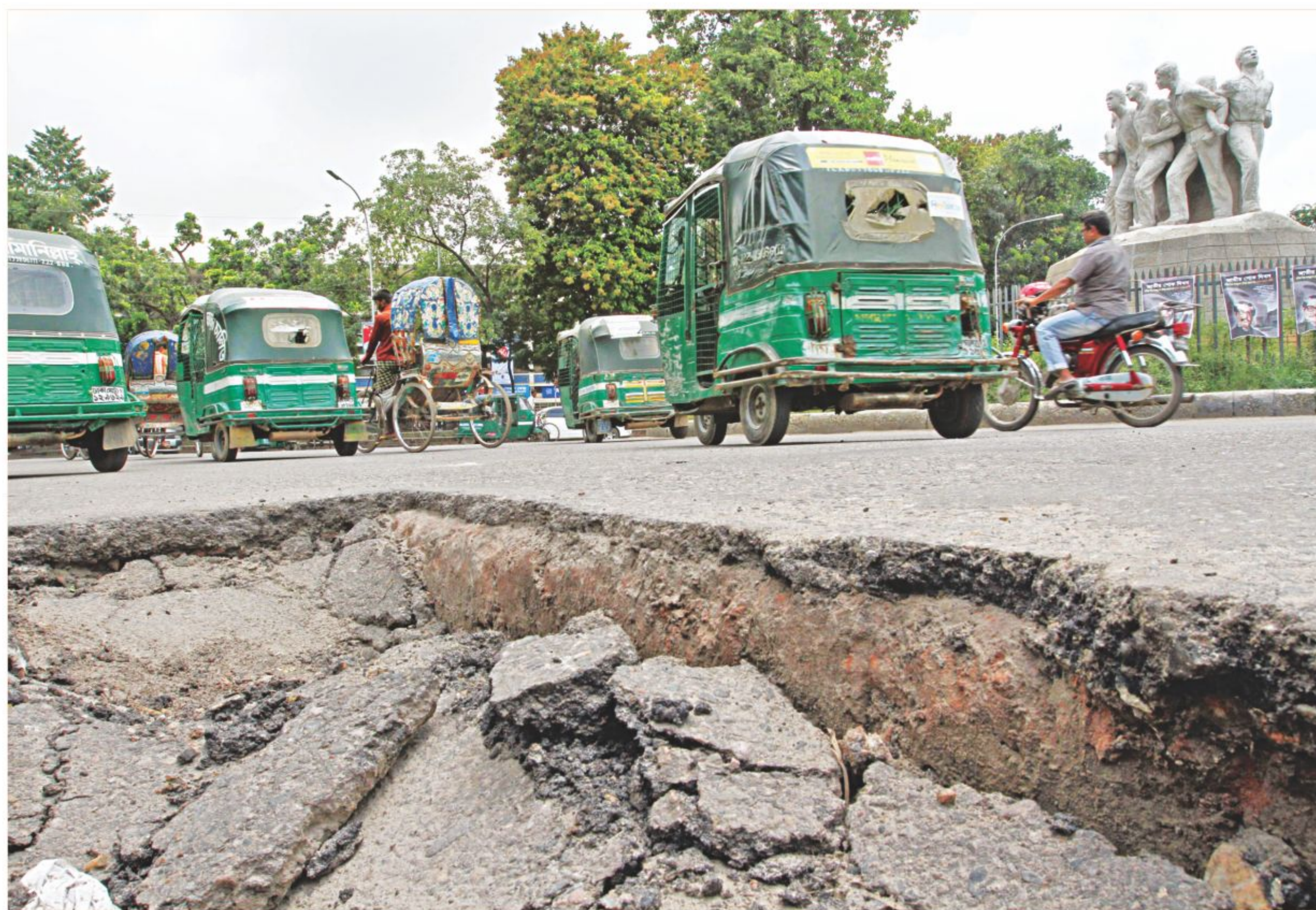
A large chunk of the road surface at TSC intersection on Dhaka University campus has sunk, posing a threat to vehicles and pedestrians. The photo was taken yesterday.
