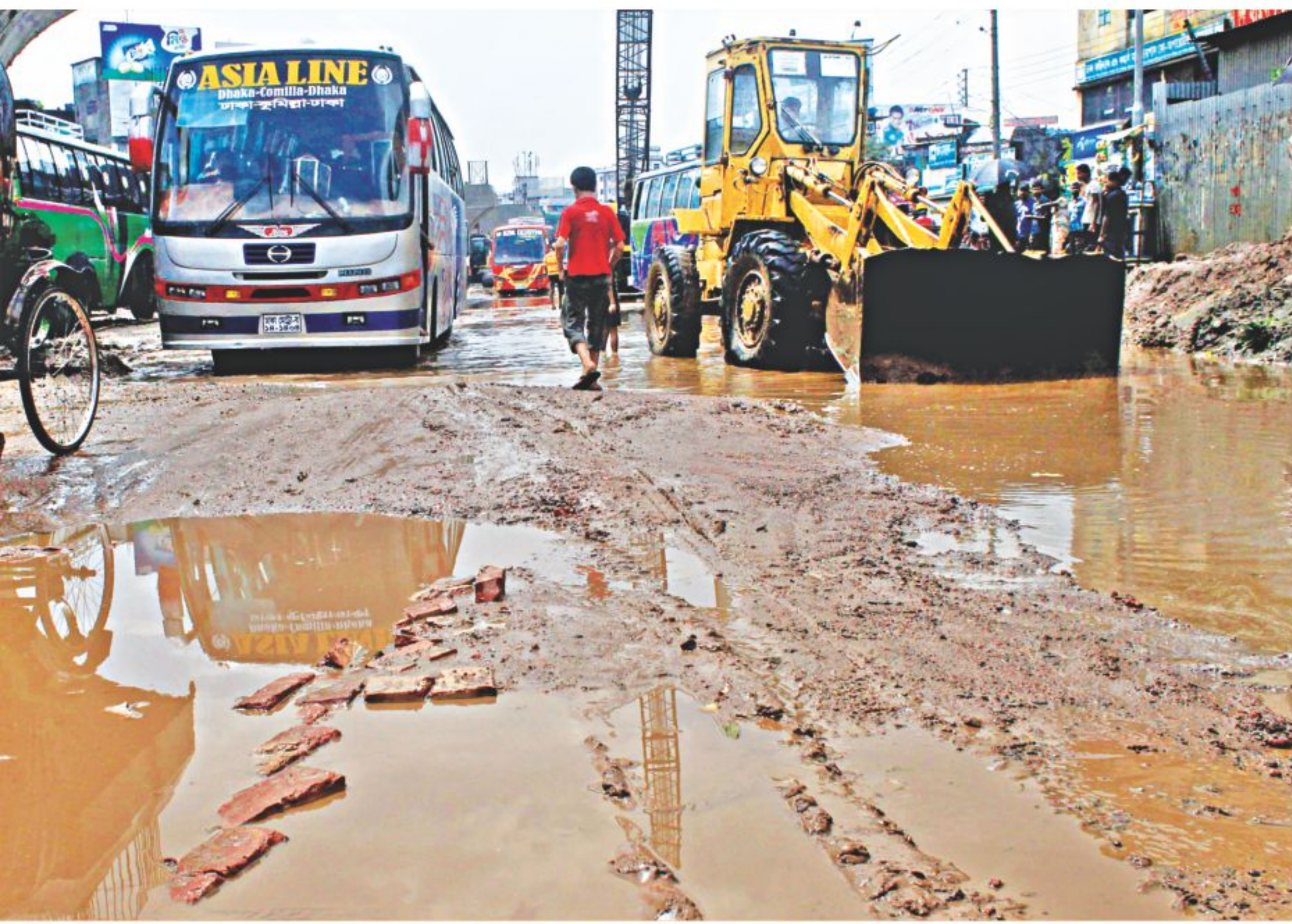
One would hardly call it a road given the condition it turned into after a brief spell of rain. The city corporation authorities were trying to restore the busy road at the capital's Sayedabad over the last two weeks, but rain has been disrupting the repair work over and over again. The photo was taken yesterday.
