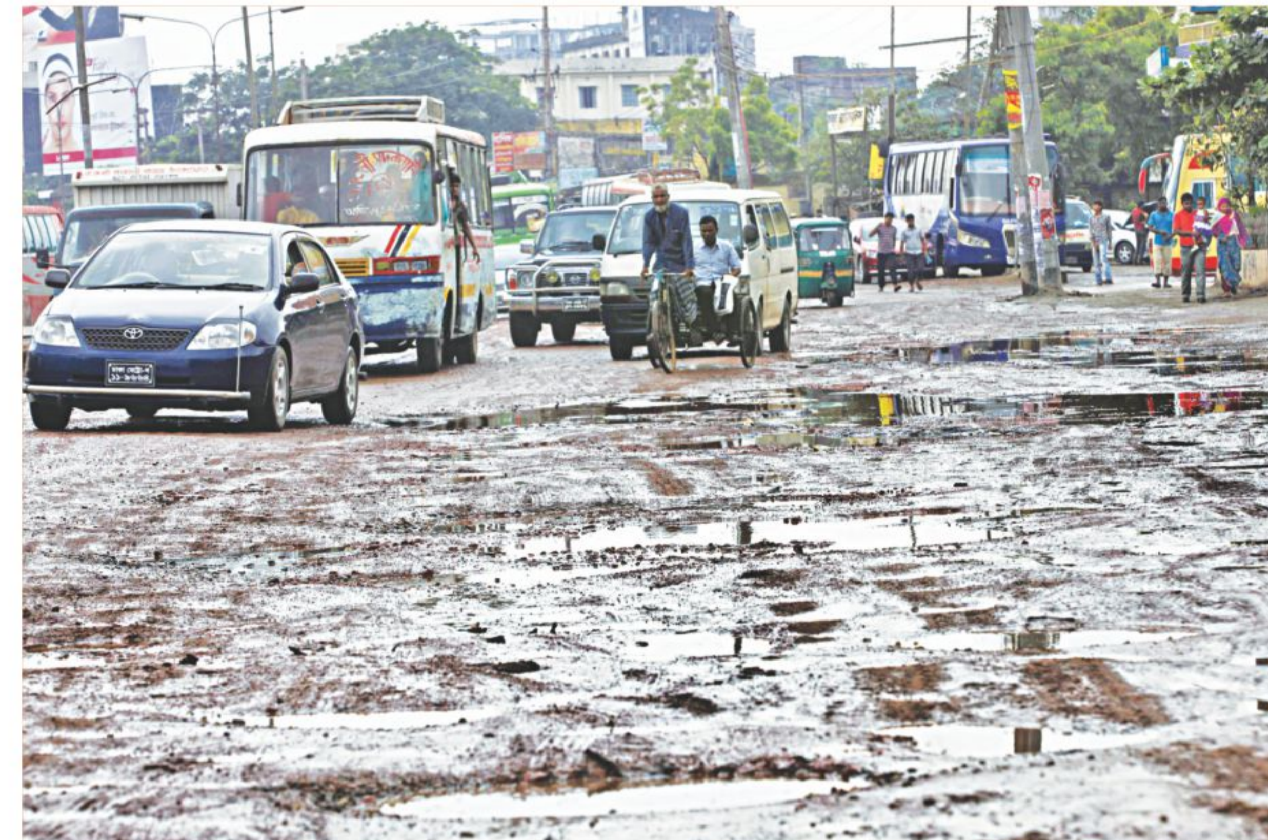
A portion of the Dhaka-Aricha highway that has been lying in a dilapidated state for a long while. Although there will be heavy traffic on this road during the Eid holidays, there has been no sign of repairing it yet. The photo was taken yesterday at Gabtoli in the capital.
