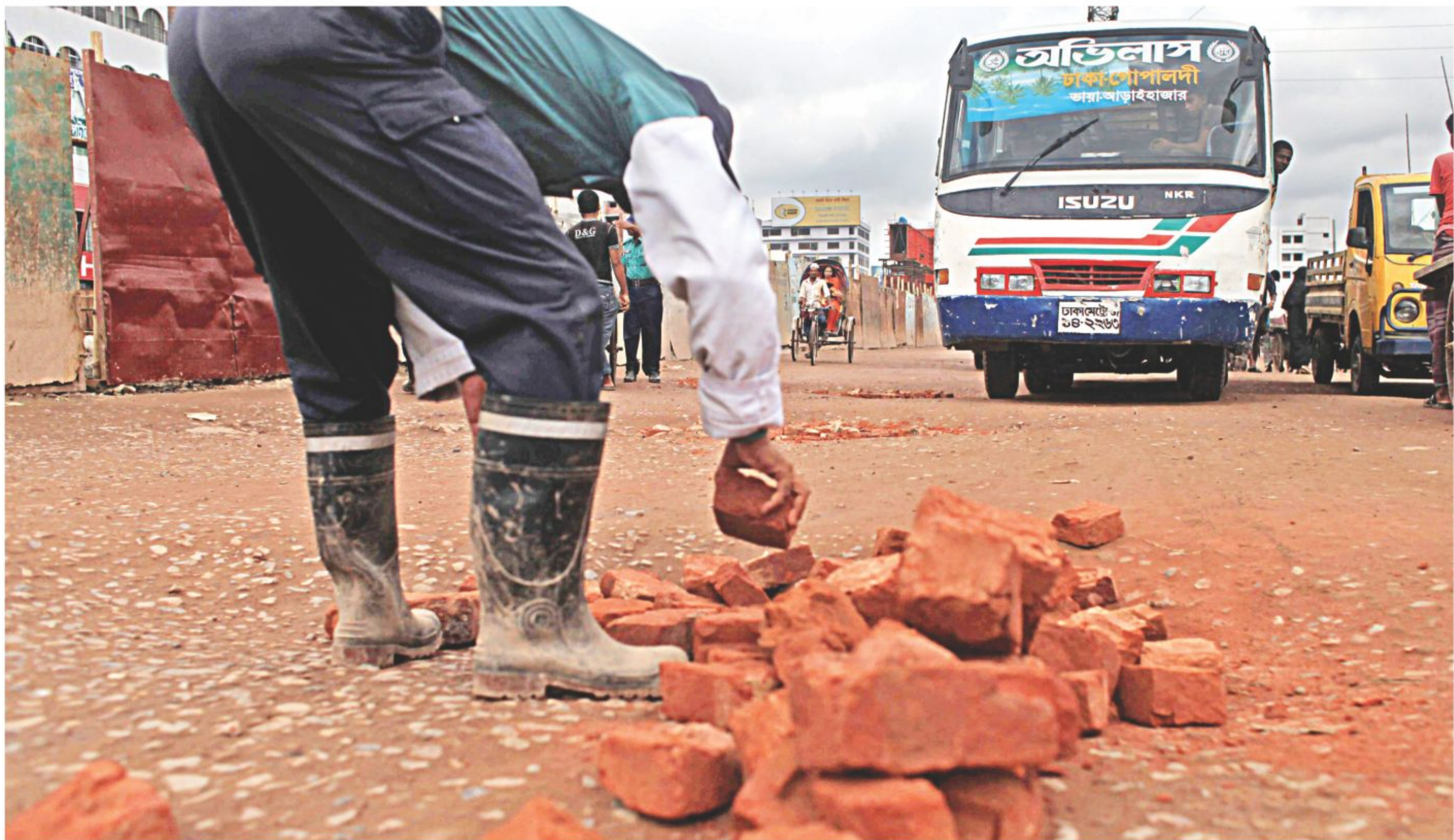
A traffic policeman tries to mend the roads with brick chips at Jatrabari in the capital. Construction of a flyover there, poor or zero road maintenance, and heavy traffic flow have left the road in tatters. A lot of people heading home for their Eid holidays would be using this road.
