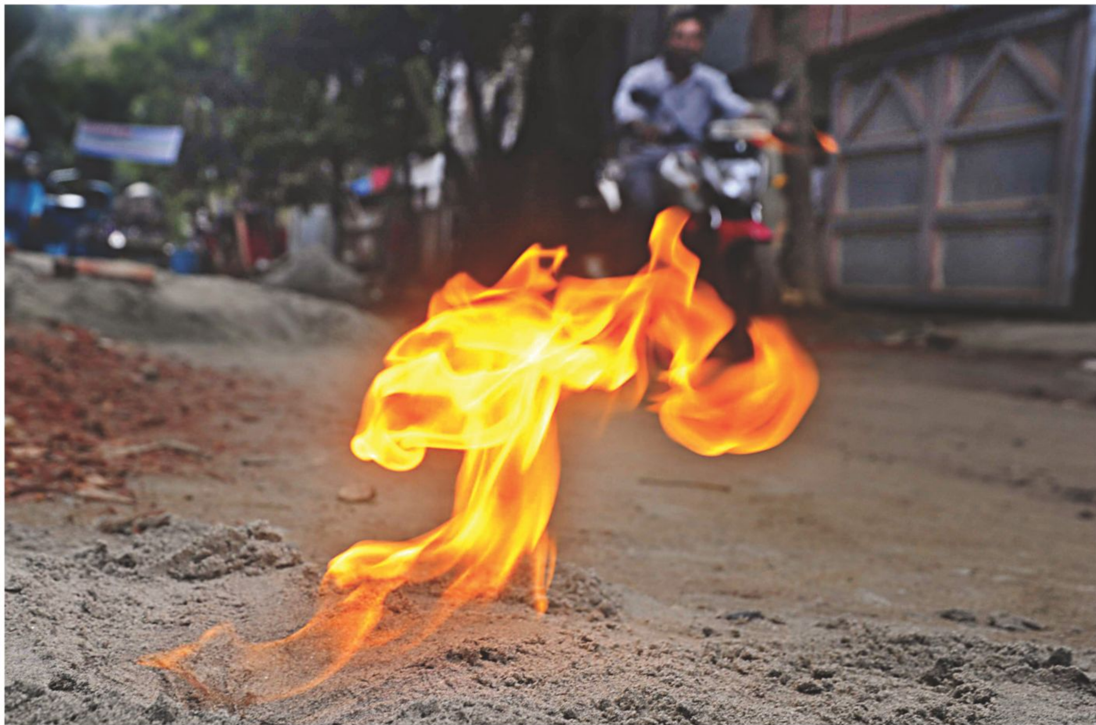
This fire on Road-7 of Block-A in the capital's Mirpur section-10 is because of leakages in the underground gas pipeline. There are at least 20-25 spots where a burning matchstick can trigger a massive fire. The photo was taken yesterday afternoon.
