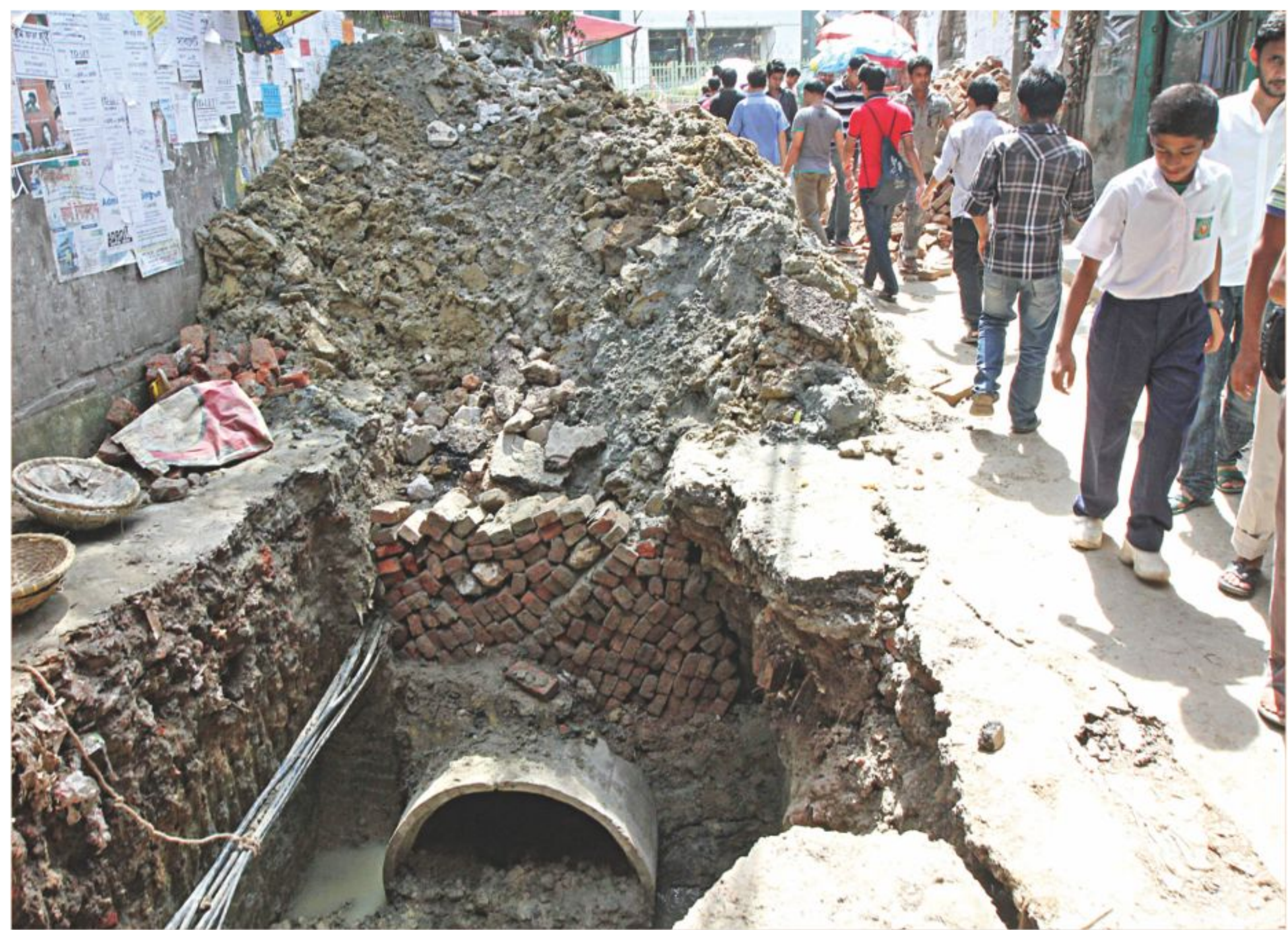
People take troubles in walking the road in the capital's Sobhanbagh neighbourhood, as it has long been left excavated for installation of sewers. The photo was taken yesterday.
