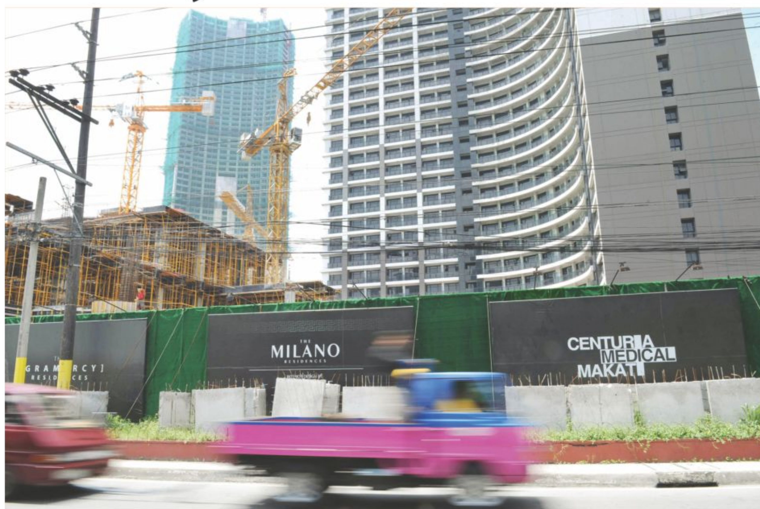
Commuters drive past a high-rise building construction site in Manila. As a Philippine property boom gathers pace, even Paris Hilton, Donald Trump and high-fashion house Versace are getting a piece of the action.
