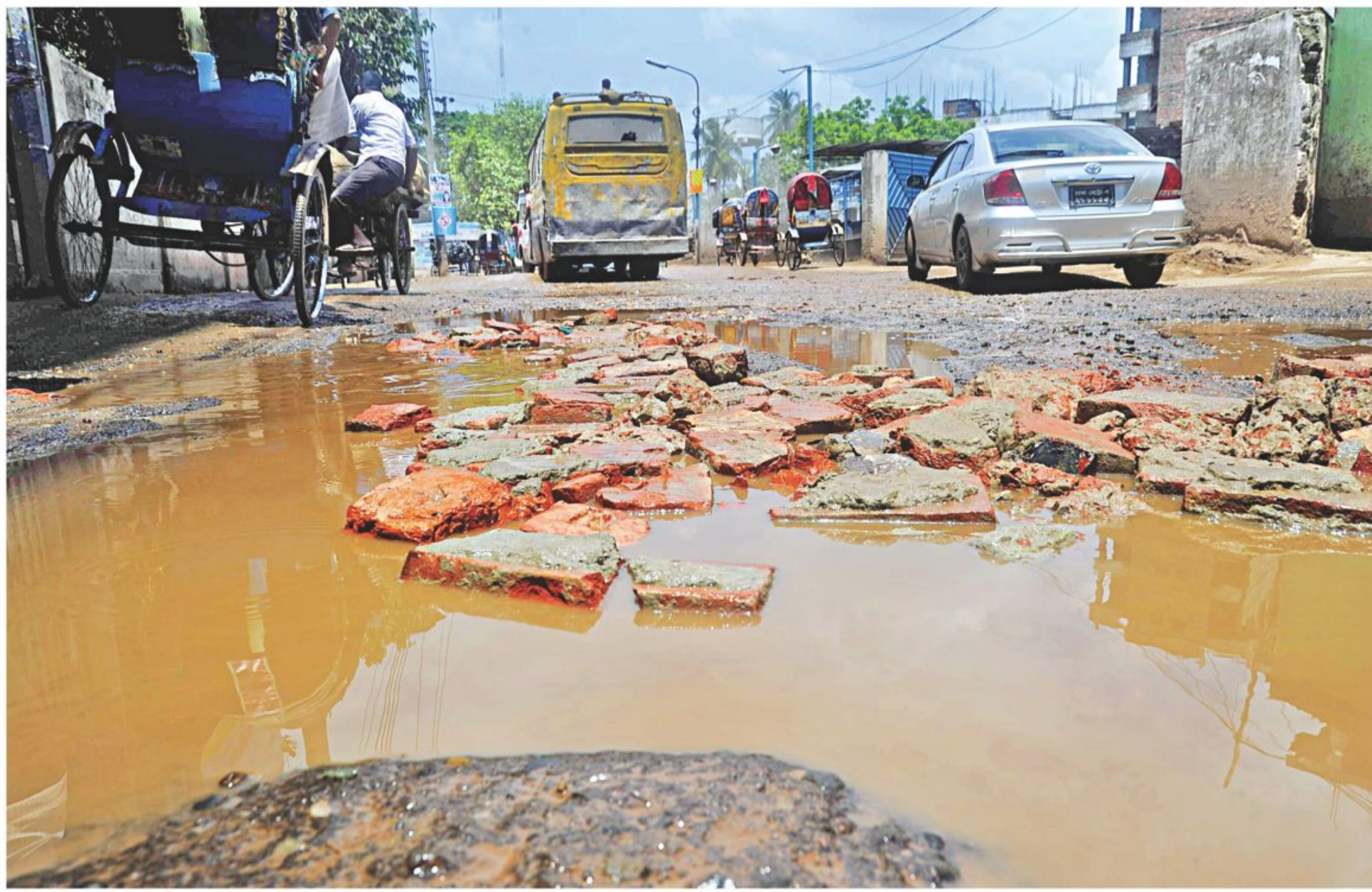
The authorities concerned have dumped rubble into potholes on Circular Road near the capital's Joykali Mandir as a stopgap solution instead of going for proper maintenance. The photo was taken yesterday.
