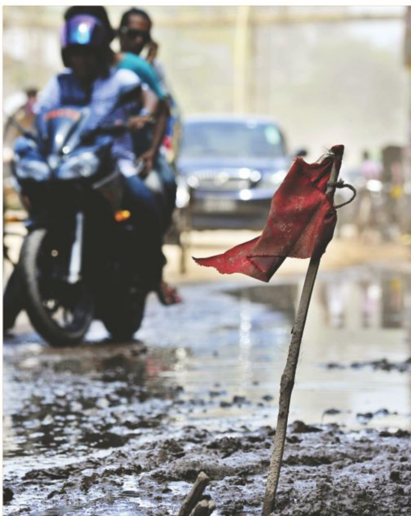
A red flag has been planted at Dayaganj intersection in the capital to warn unwary vehicles and commuters of an open man-hole hidden amidst the mud and dirt on the road.
