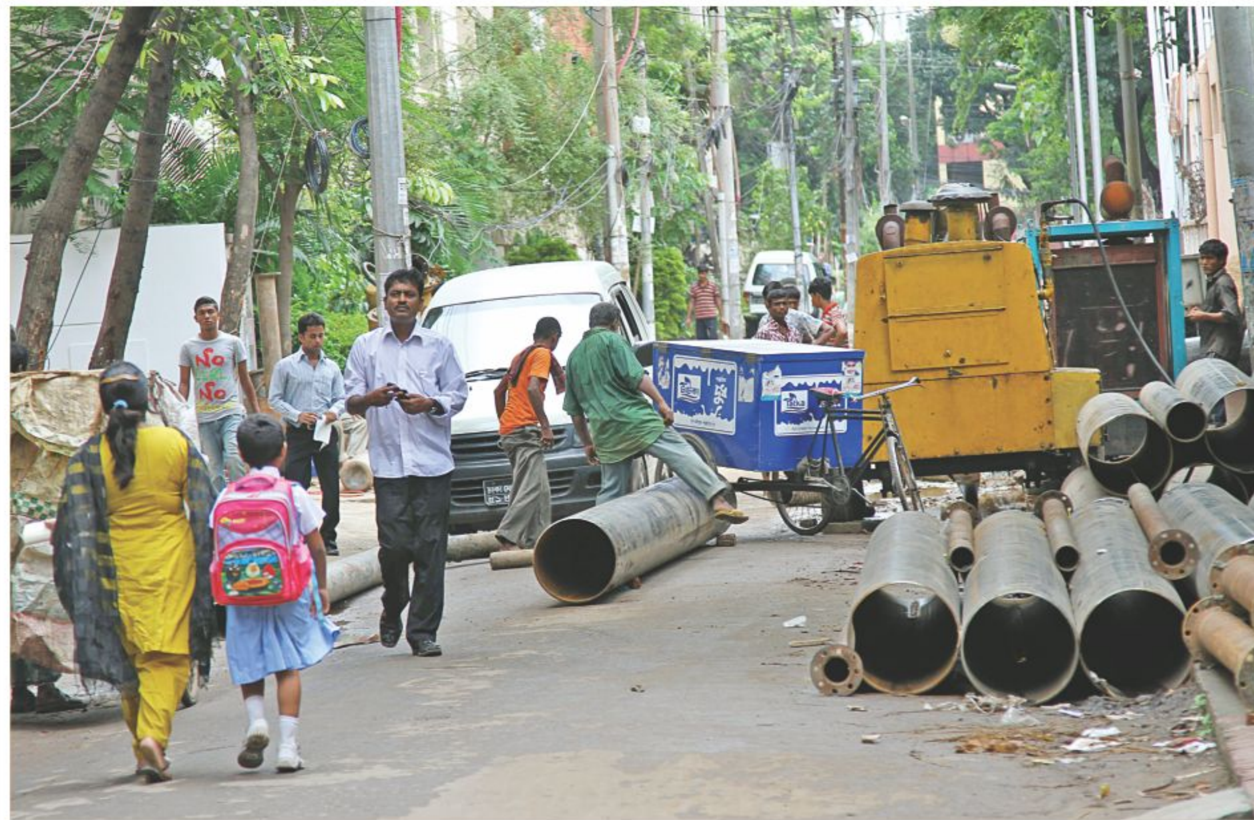
Workers of Dhaka Wasa almost close off Road-13/A Dhanmondi in the capital yesterday to install a deep tube well nearby, much to the dismay of the locals.
