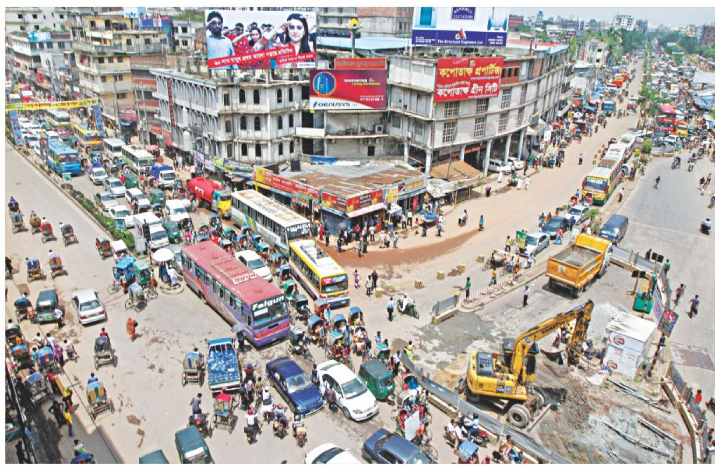
Roads of Khilgaon, Mouchak and Rampura adjacent to Malibagh level crossing witness traffic jam all day long due to digging at the intersection as a part of development project. The photo was taken yesterday.
