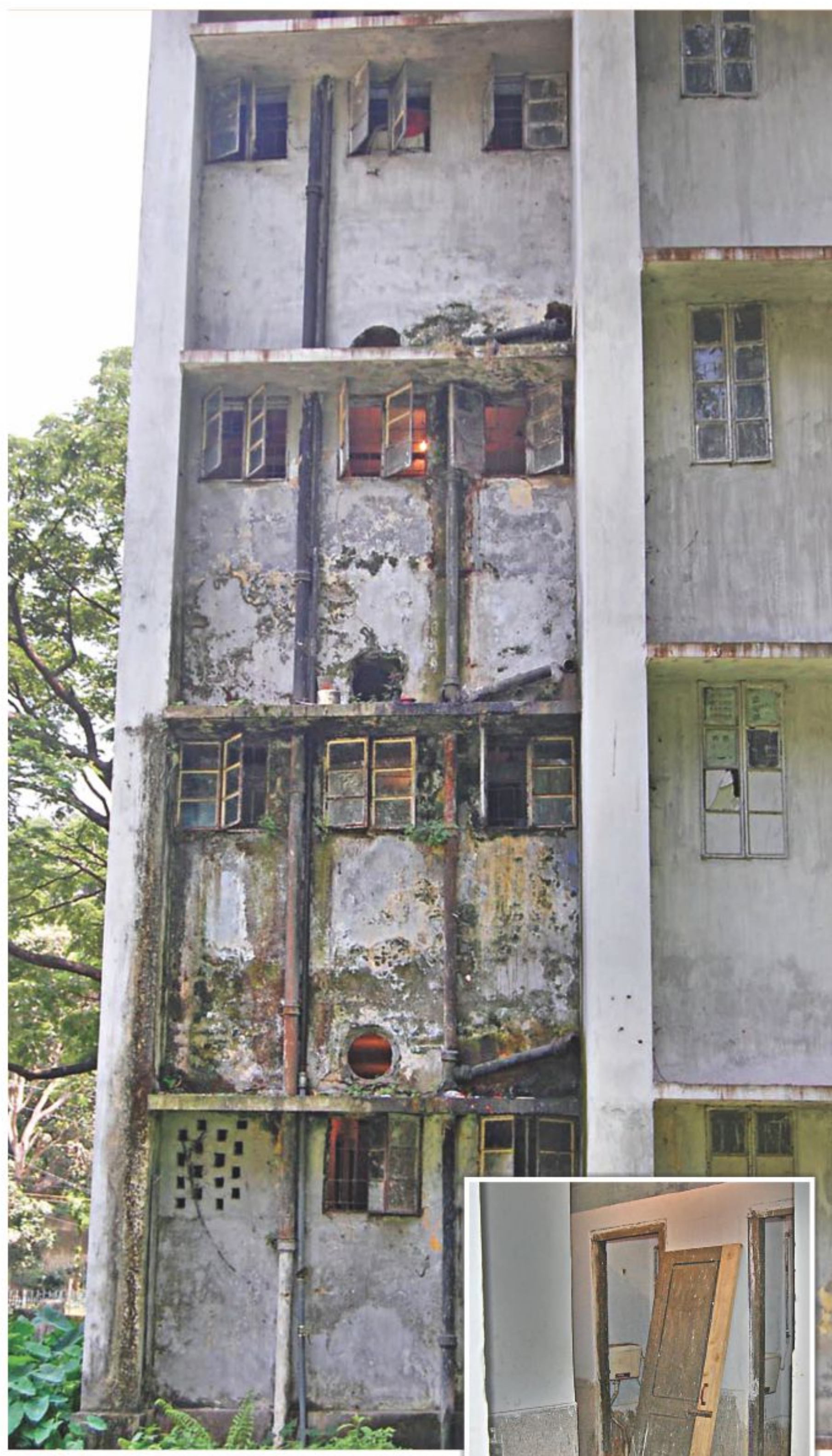
The main hostel for males of Chittagong Medical College is in a decrepit condition. (Inset) The doors of the bathrooms and toilets are unhinged with sanitary pipes leaking overhead.
