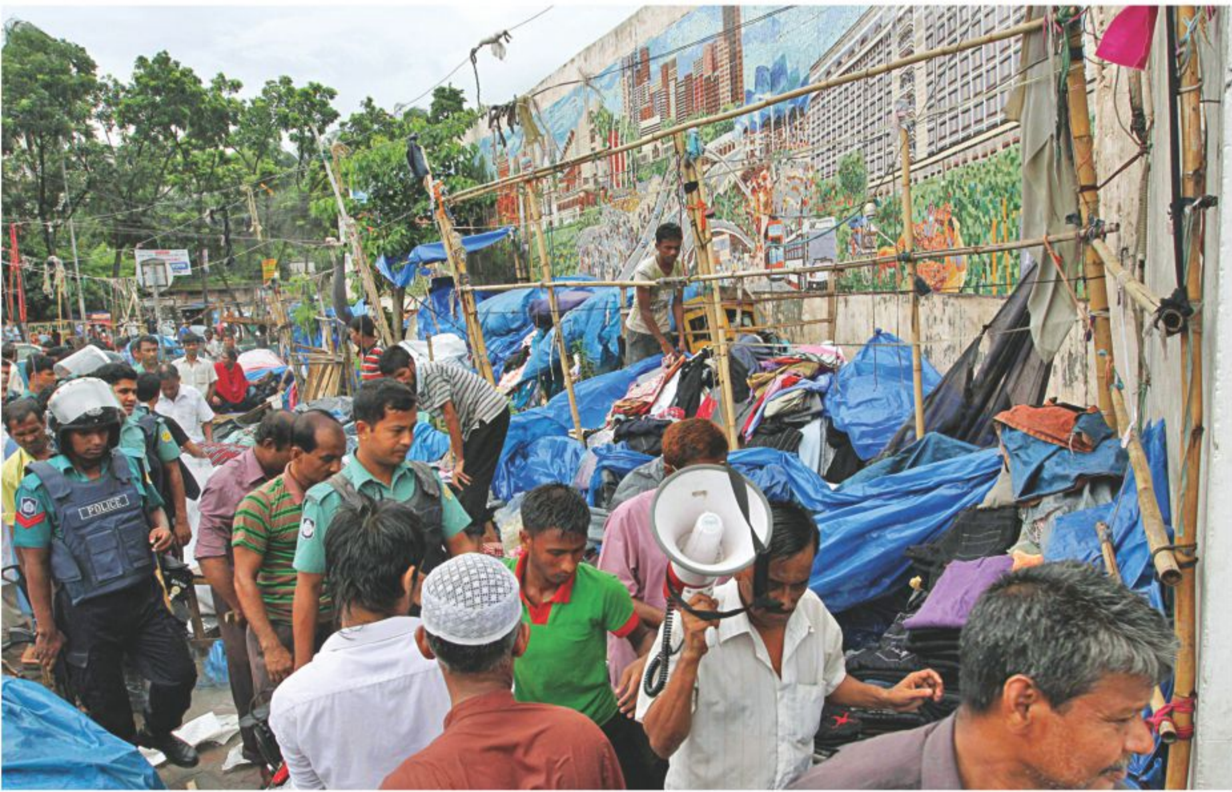
The Dhaka City Corporation (DCC) authorities demolish illegal structures on the pavement adjacent to New Market in the capital yesterday. The DCC made the move following a report in The Daily Star on Thursday.
