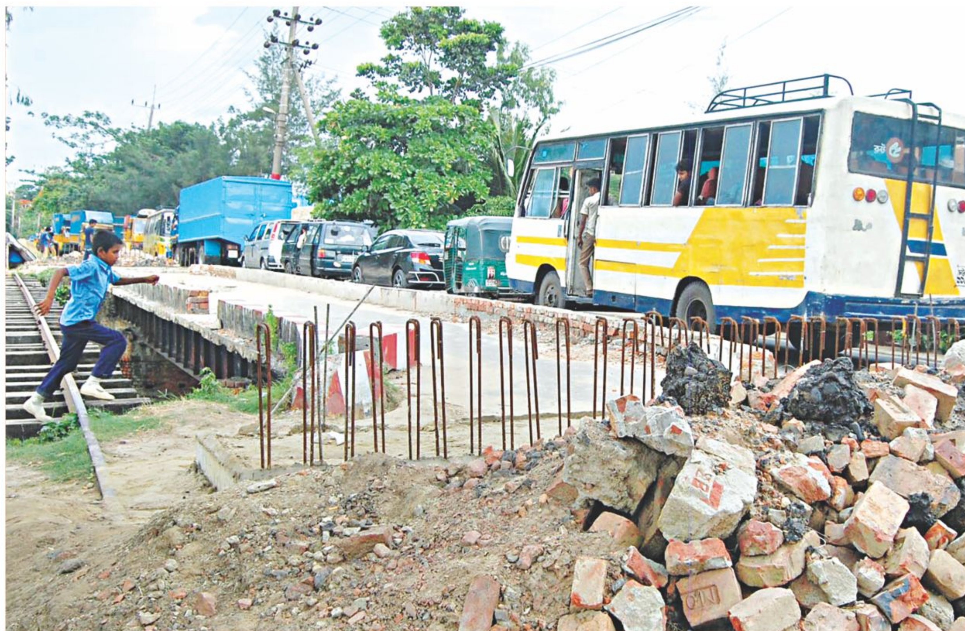
Vehicular movement narrows down to only one lane on this bridge on Patenga No 9 Pool area in Chittagong city as its repair works has been ongoing for the past seven months. The photo was taken yesterday.
