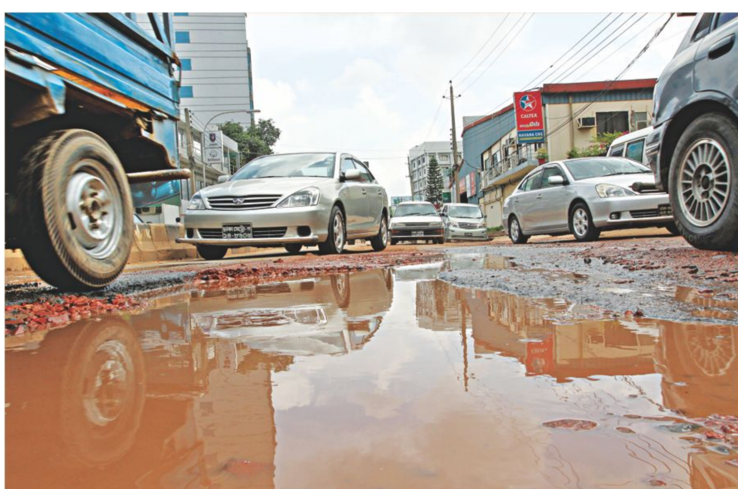
A portion of the Gulshan-Tejgaon link road lies in a dilapidated state with a big puddle in the centre, hampering the movement of vehicles on the road. The photo was taken at GMG intersection in the capital yesterday. PHOTO: PALASH KHAN
