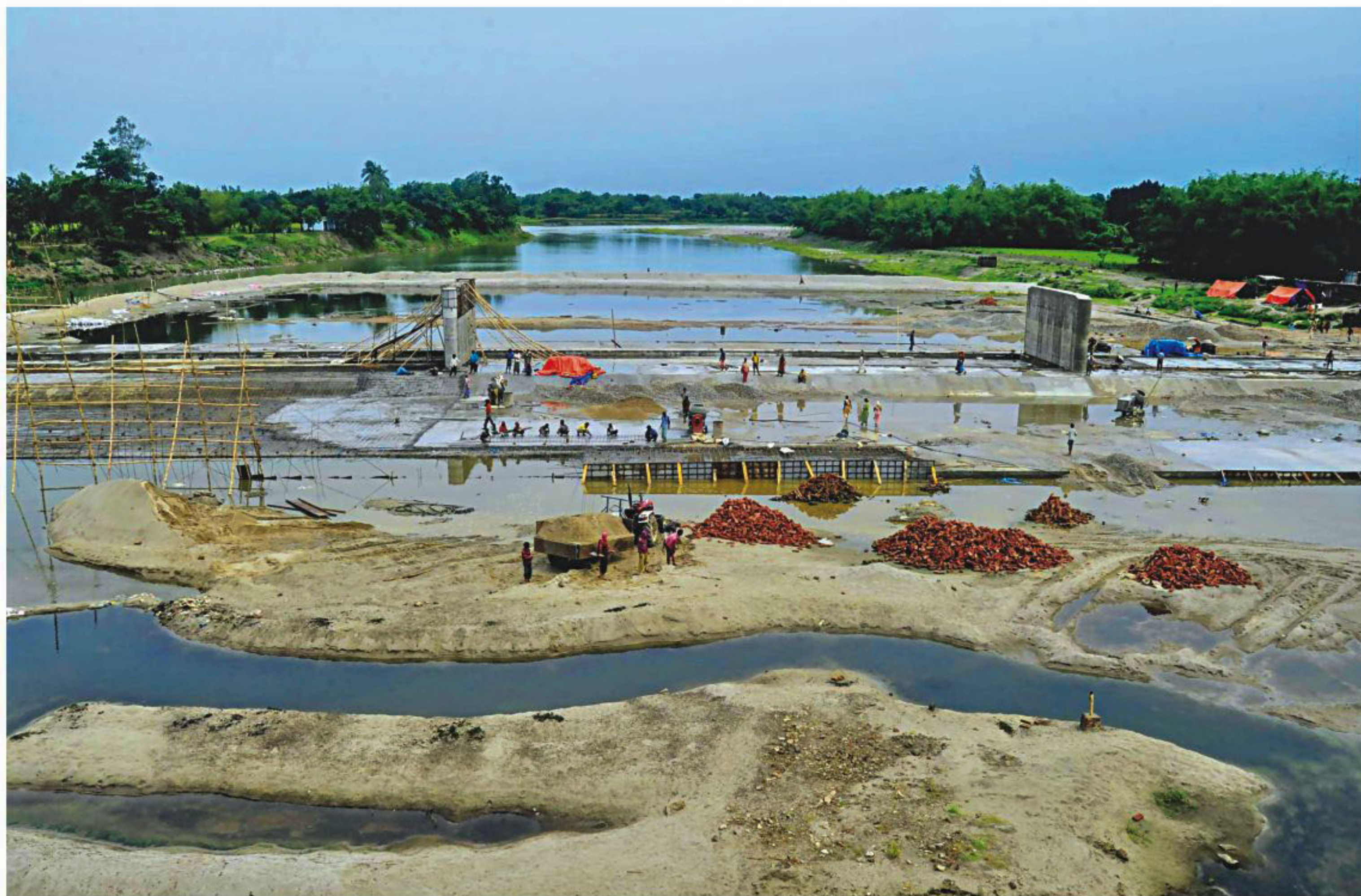
A rubber dam is being built on the Atrai in Dinajpur to create a reservoir in the river that usually dries up in the lean season. The photo was shot last week.
