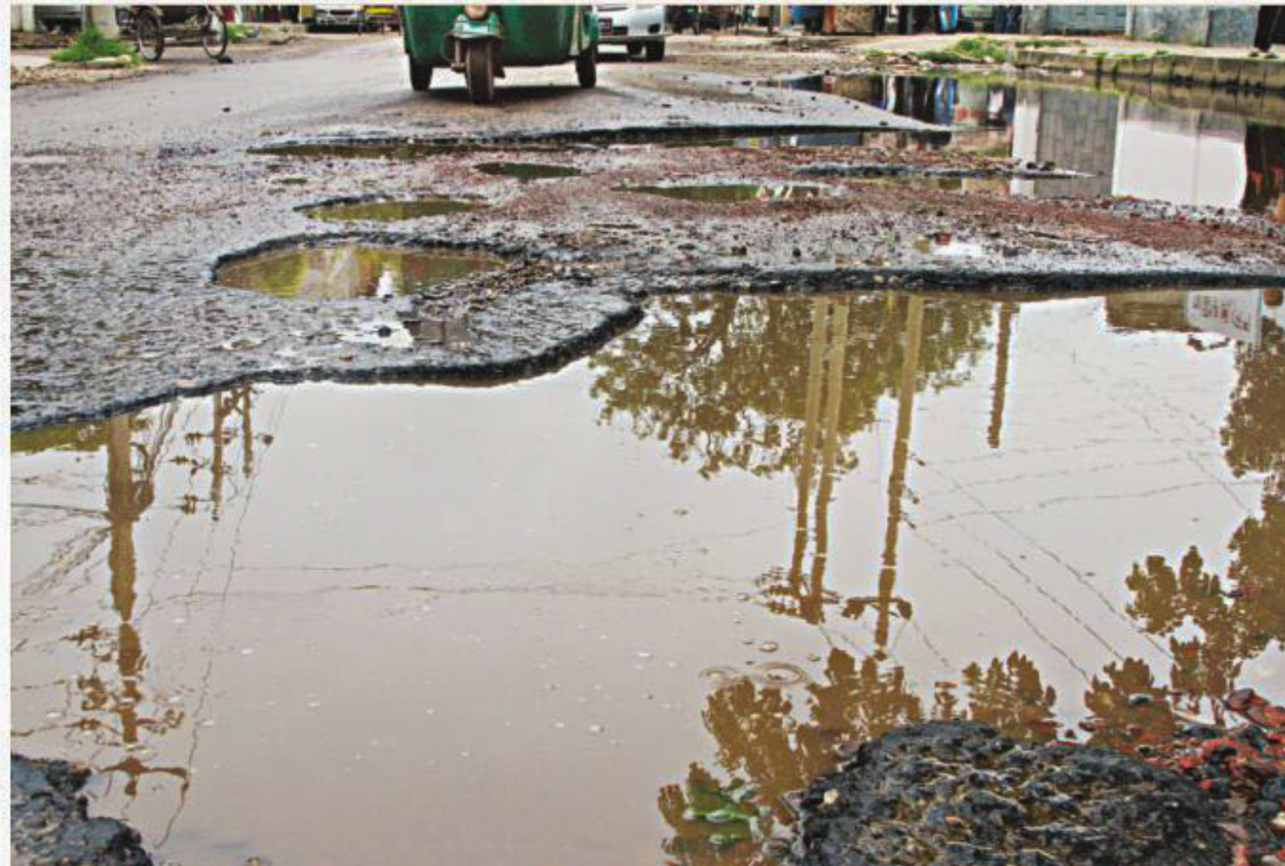
This pothole riddled road near Community Centre Adarsha High School in Tejgaon Industrial Area in the capital has been in the sorry state for quite sometime. The photo was taken recently.
