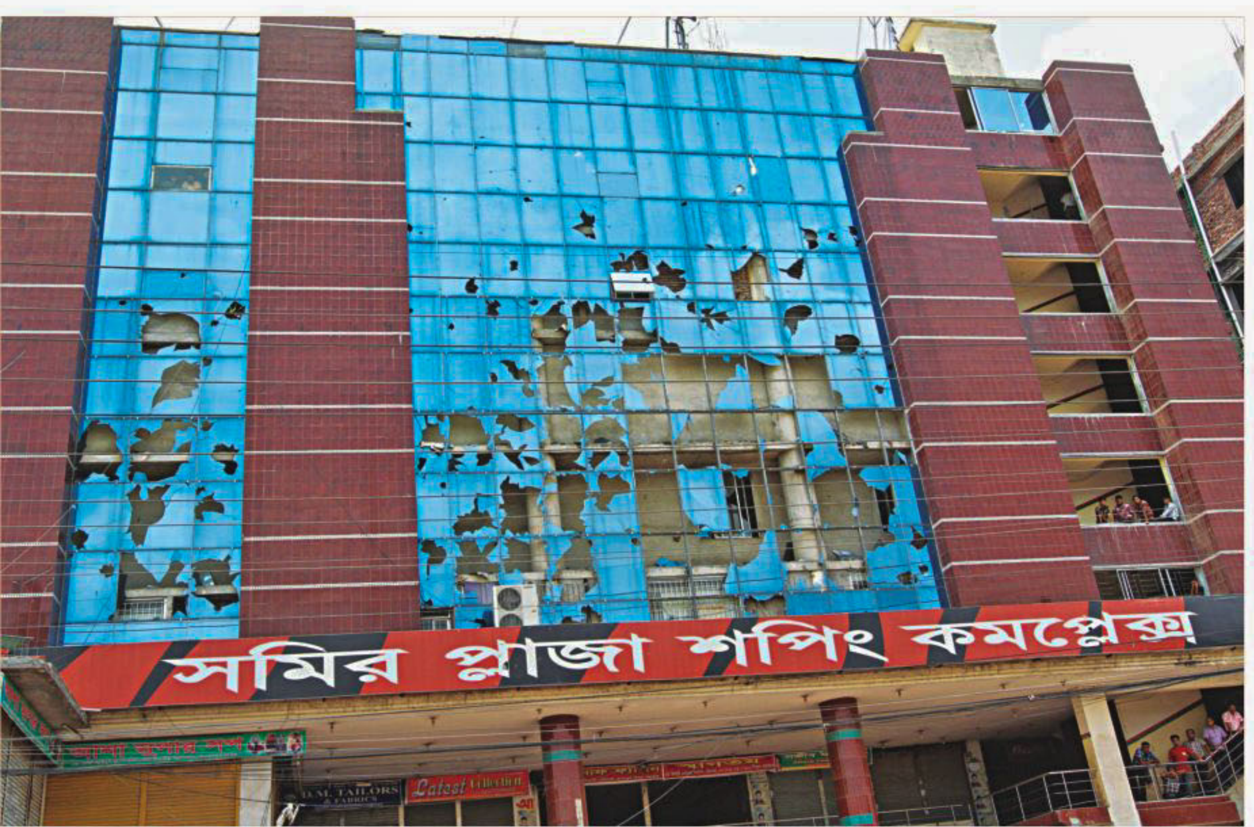
THE WRATH OF ANGRY WORKERS: A building comes under attack from protesters in the industrial hub of Ashulia on the outskirts of Dhaka yesterday. Angry garment workers staged street protests demanding a pay hike for the fourth day. Related story on page 1
