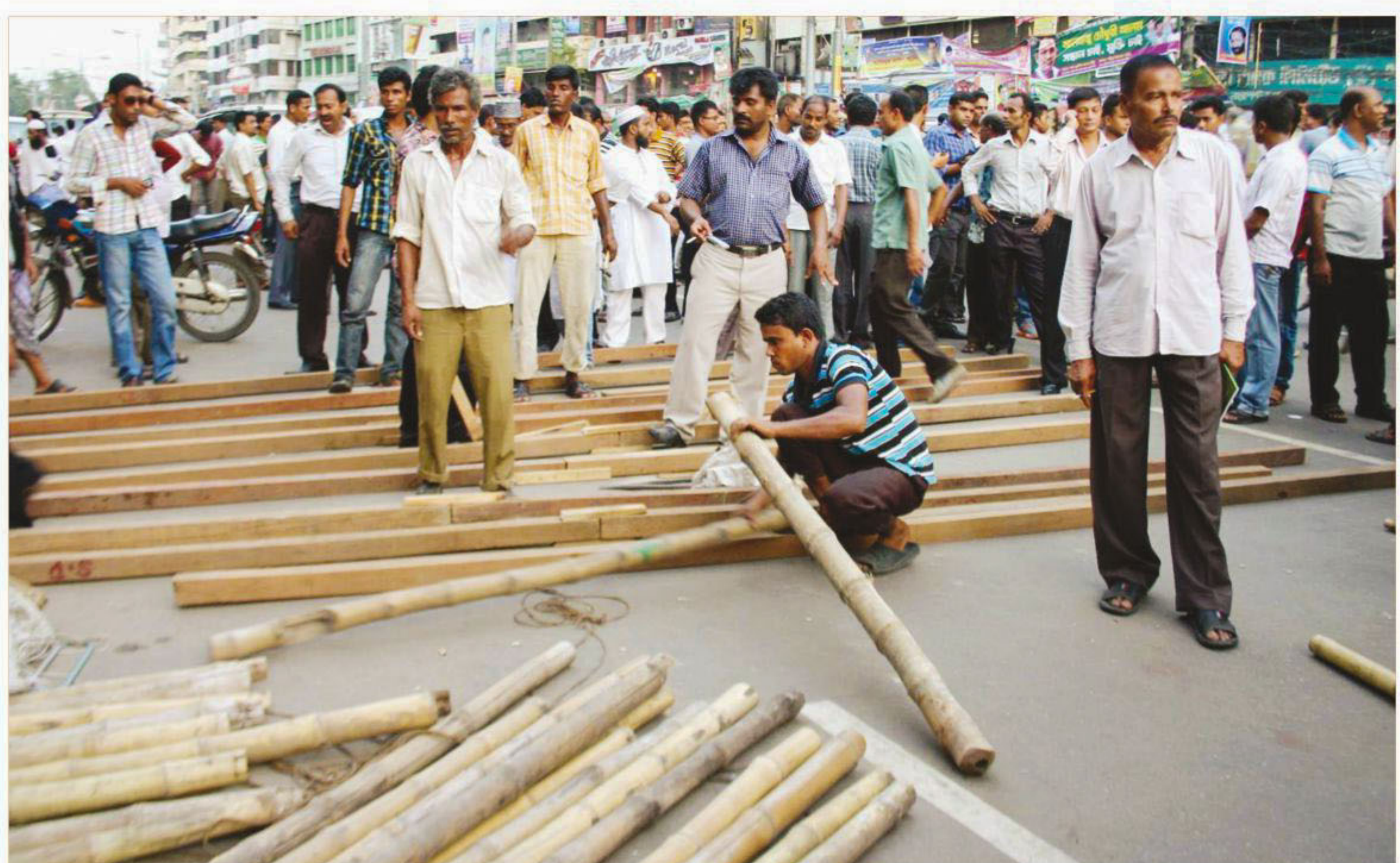
Workers constructing a stage before BNP's Naya Paltan office in the capital yesterday. The BNP-led 18-party alliance is scheduled to hold a rally here today to declare its next course of agitation programmes demanding restoration of the caretaker government system.
