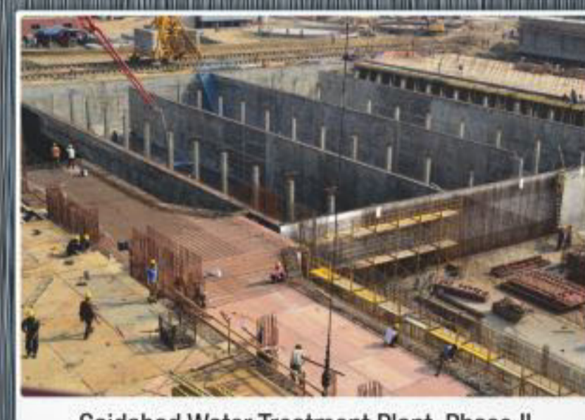
Saidabad Water Treatment Plant, Phase II
