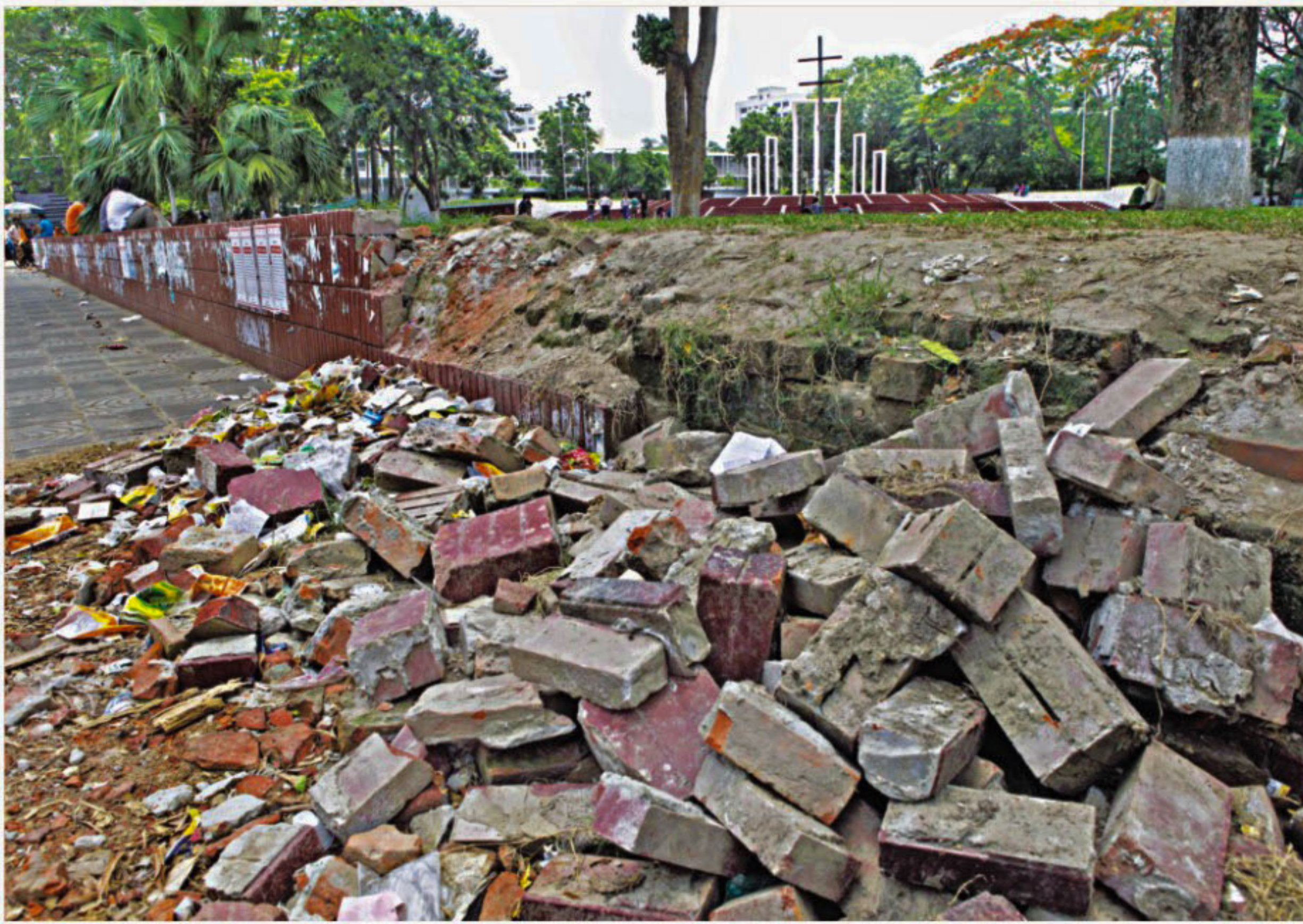
The Central Shaheed Minar boundary wall, which crumbled after a tree branch fell onto it, fails to grab the attention of the authorities even a week into the incident. The photo was taken yesterday.
