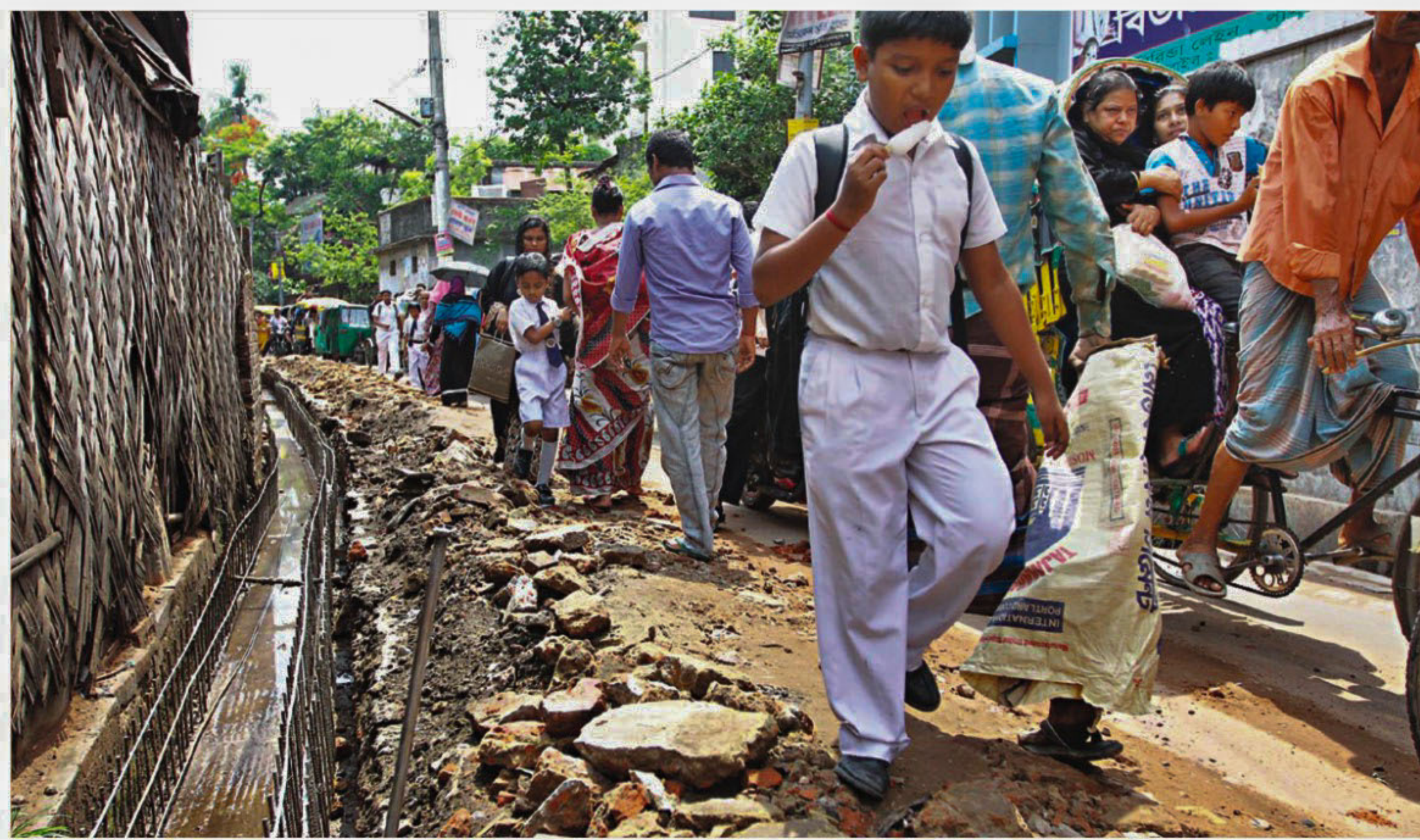
A school boy walks by gravel, mud and construction materials piled up on Mirinda Lane at Pathorghata in Chittagong as part of repair works of a drain on the lane. The repair work, which was undertaken by Chittagong City Corporation, was ongoing for more than 20 days, causing huge sufferings to pedestrians and commuters in the area. The photo was taken recently.
