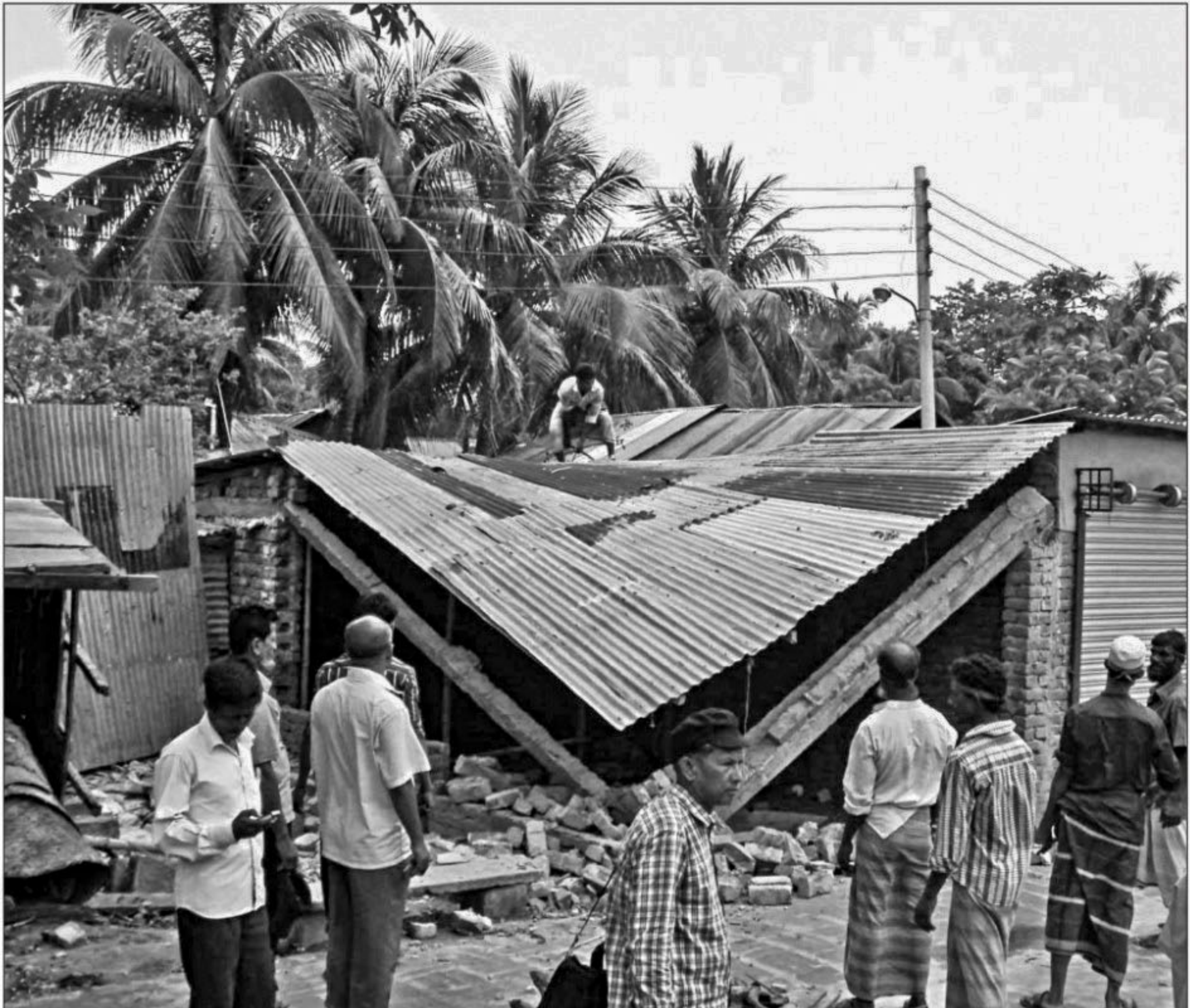
PHOTO: STAR Authorities demolish illegally erected structures on the land of Bangladesh Railway in Chandpur town yesterday.
