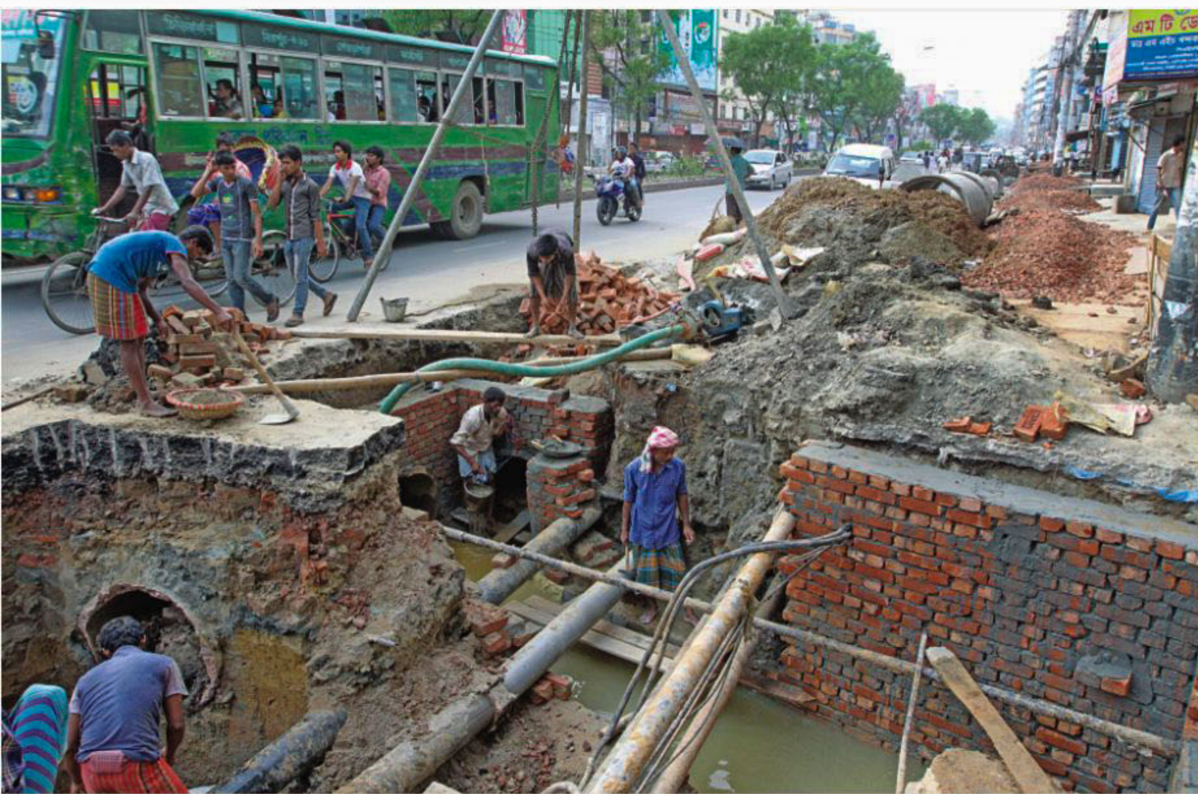
PHOTO: STAR Only a small number of workers, appointed by Dhaka Wasa, work to install sewage pipes on Begum Rokeya Sarani in the capital, lengthening the duration of work and causing suffering to passers-by. The photo was taken yesterday.
