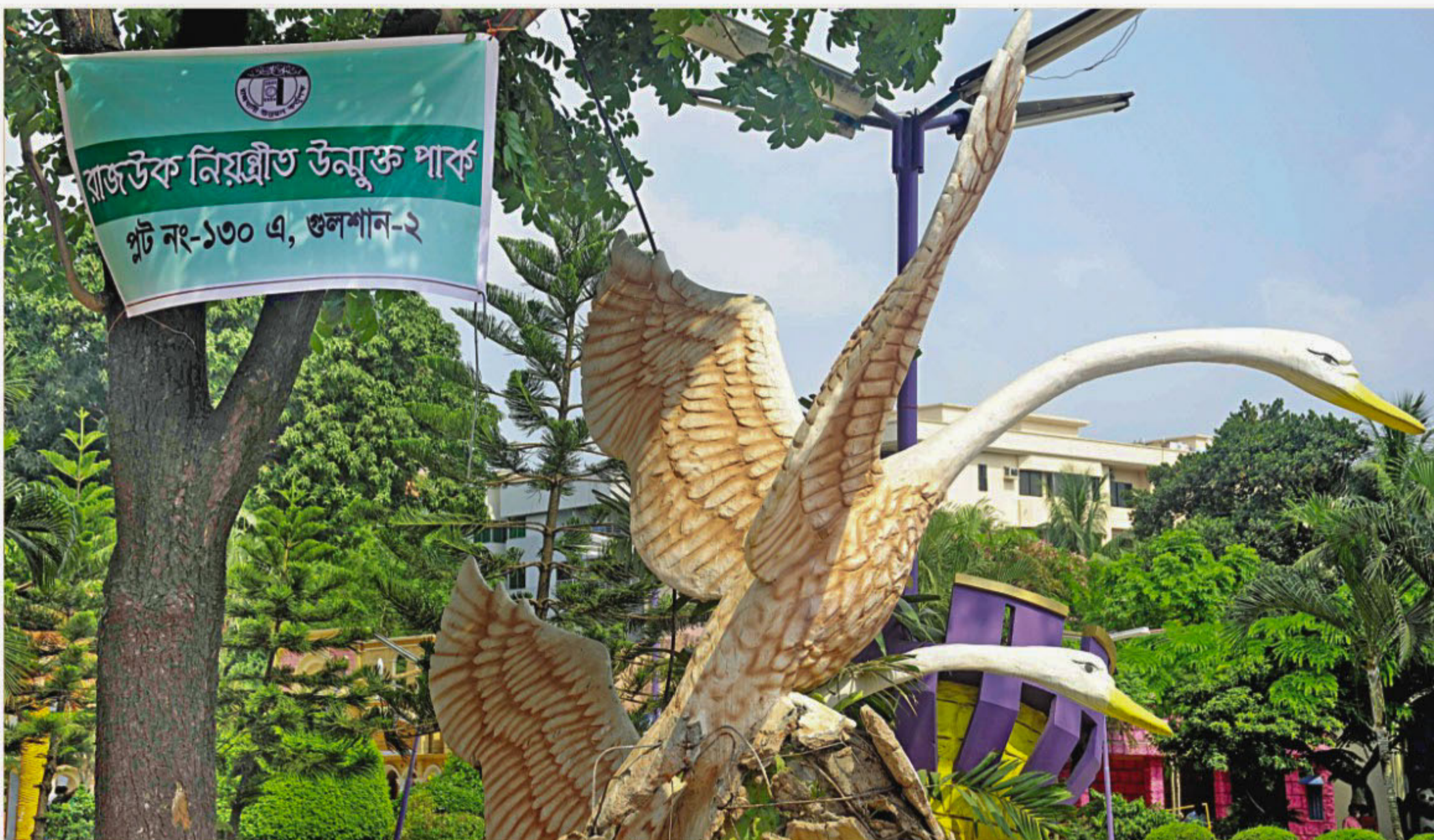
Rajdhani Unnayan Kartripakkha (Rajuk) hangs up a notice yesterday declaring the plot, once housing Wonderland amusement park, as a public park of the capital. Rajuk demolished the main entrance and boundary wall of the park on Monday to free around four acres of land of Gulshan central playground following what they said was a Supreme Court verdict.
