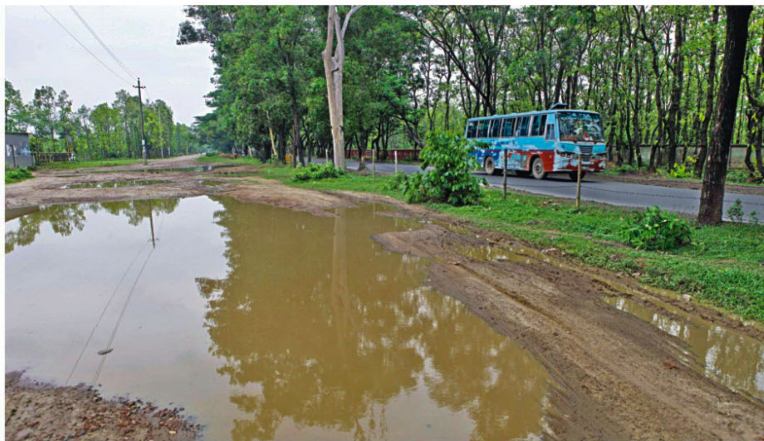
A section of Dhaka-Mymensingh highway is in tatters. The progress of upgrading the road into a dual carriageway is at snail's pace as the government and the contractor concerned play the blame game. The photo was taken from Rajendrapur, Gazipur.
