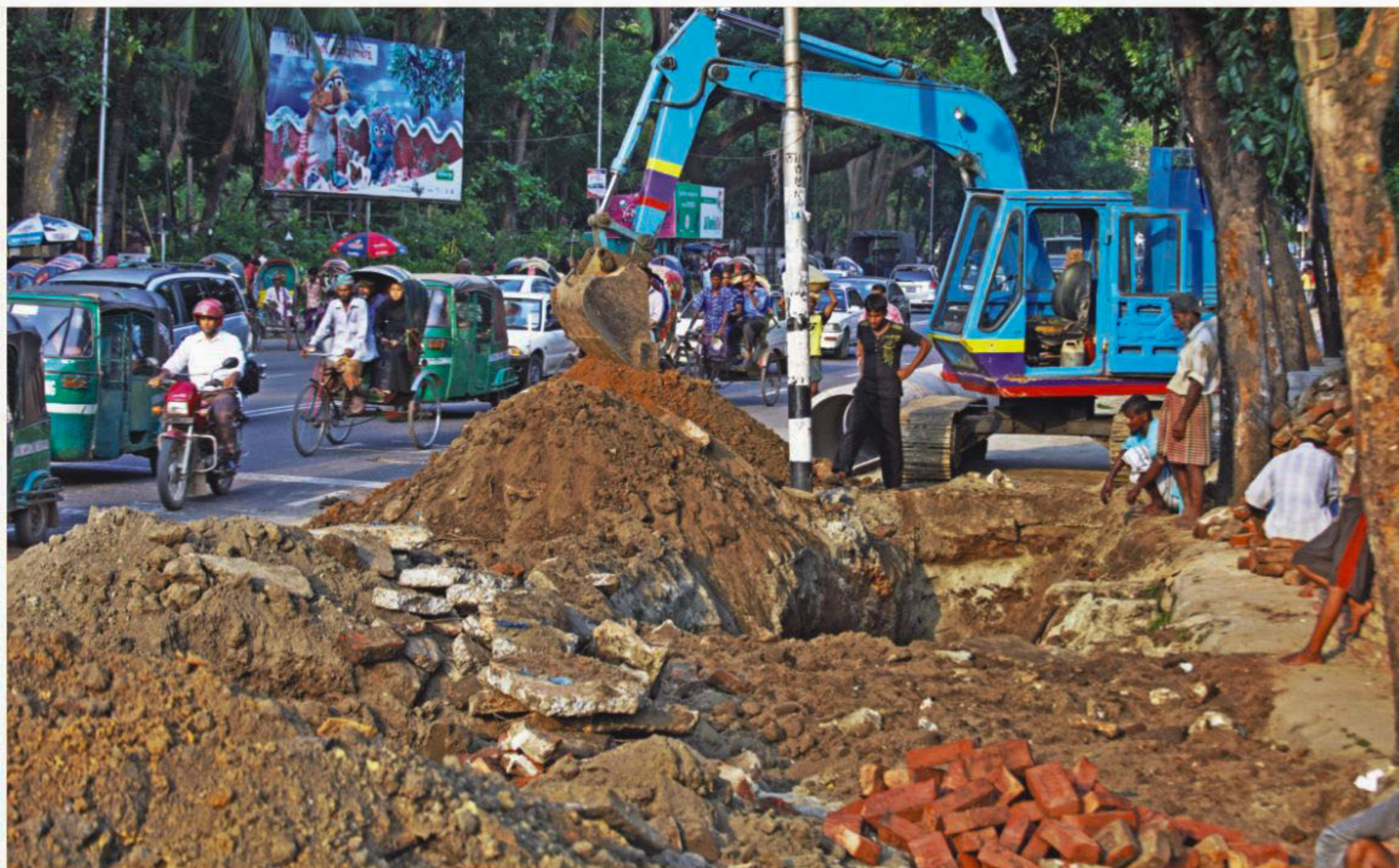
Pedestrians' suffering increases due to Dhaka City Corporation's (DCC) long-drawn development work on the footpath in front of Curzon Hall at Dhaka University. The photo was taken yesterday.
