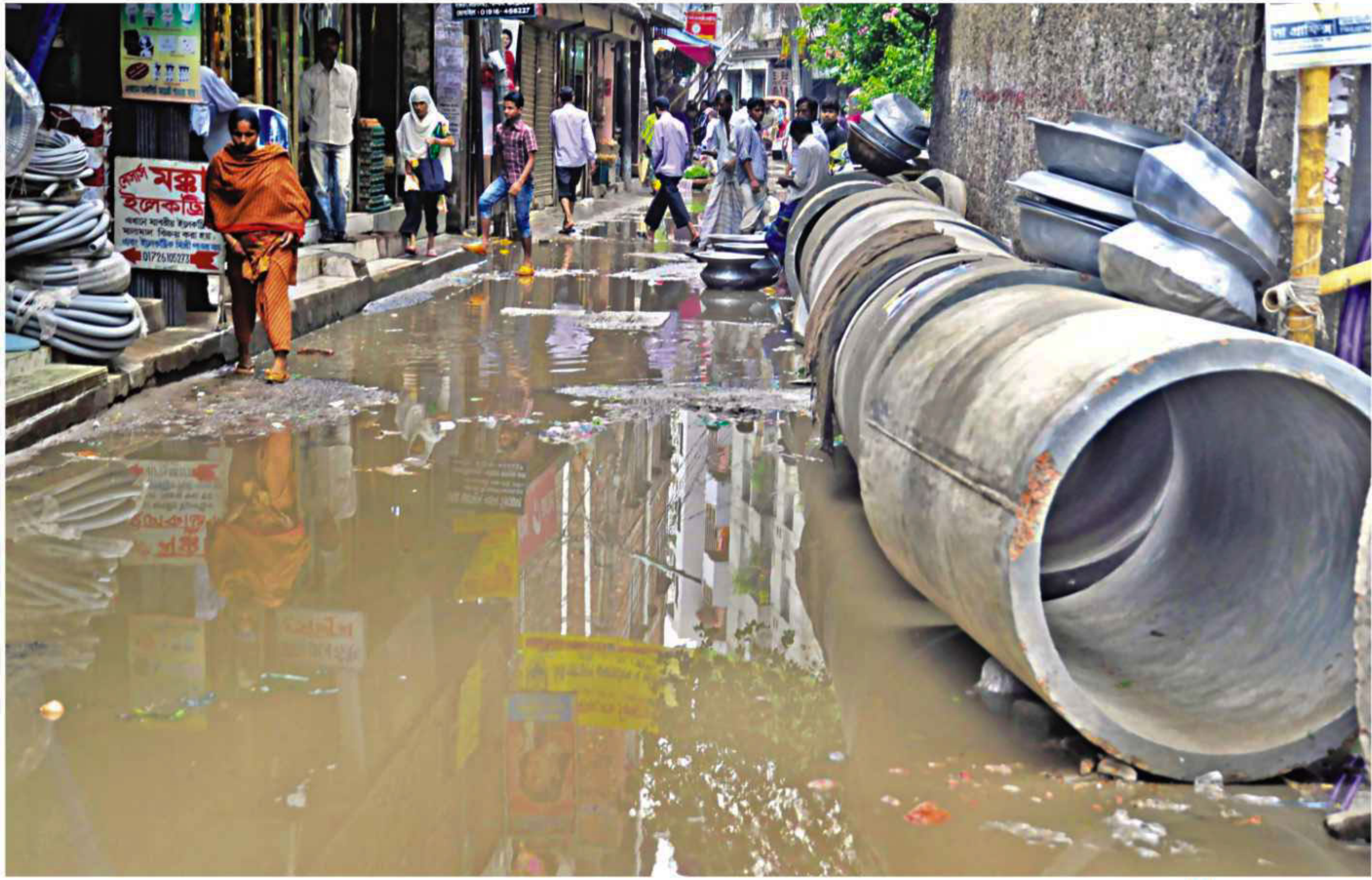
The DIT Road at the capital's Rampura is in bad shape and needs immediate repair. Whenever it rains, water accumulates in potholes of the road, which is also narrowed with sewerage pipes waiting to be installed. The photo was shot recently.
