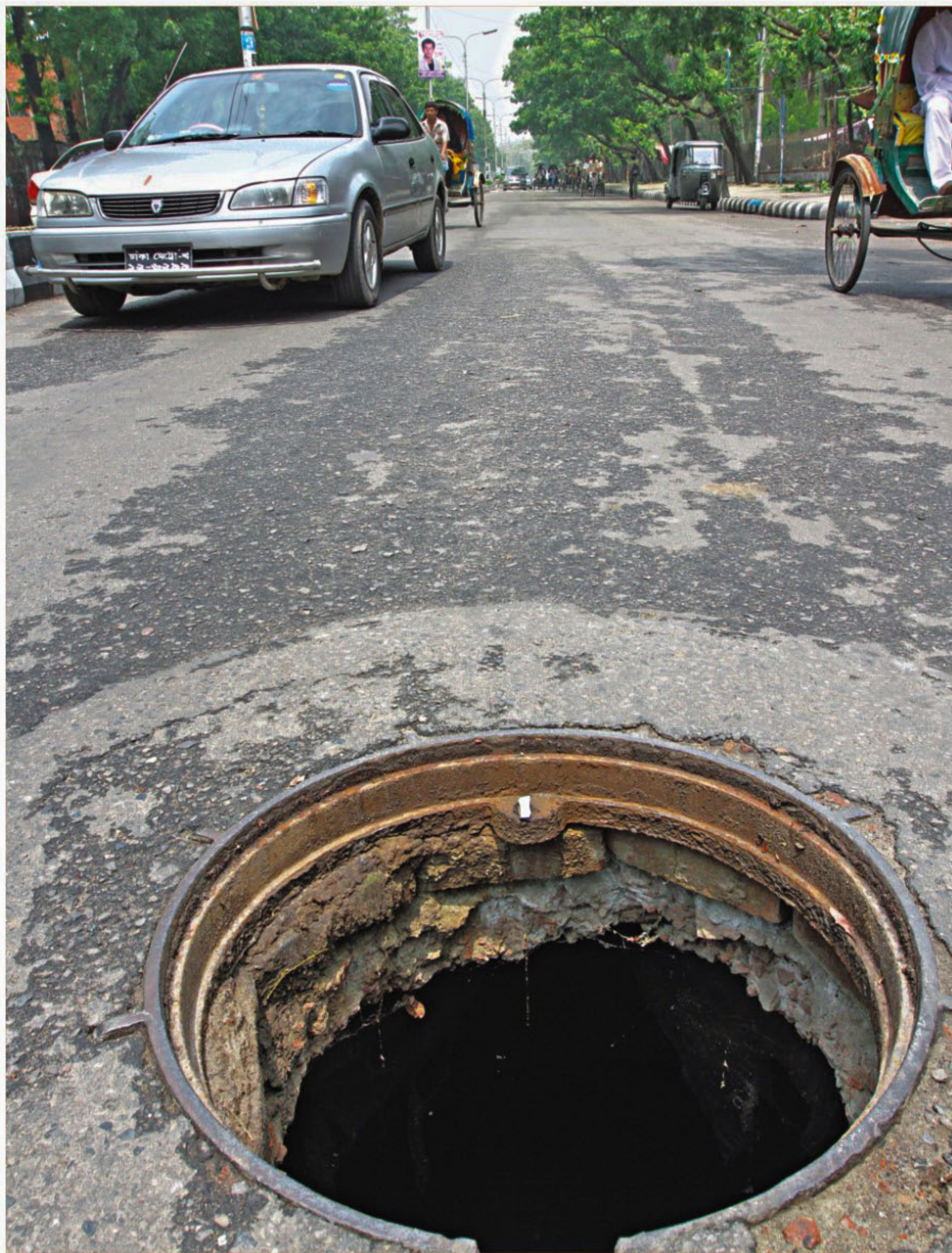
A manhole sans lid before the capital's Bangla Academy, the very road over which the celebratory procession marking Pehela Baishakh will pass tomorrow. The photo was taken yesterday. PHOTO: PALASH KHAN
