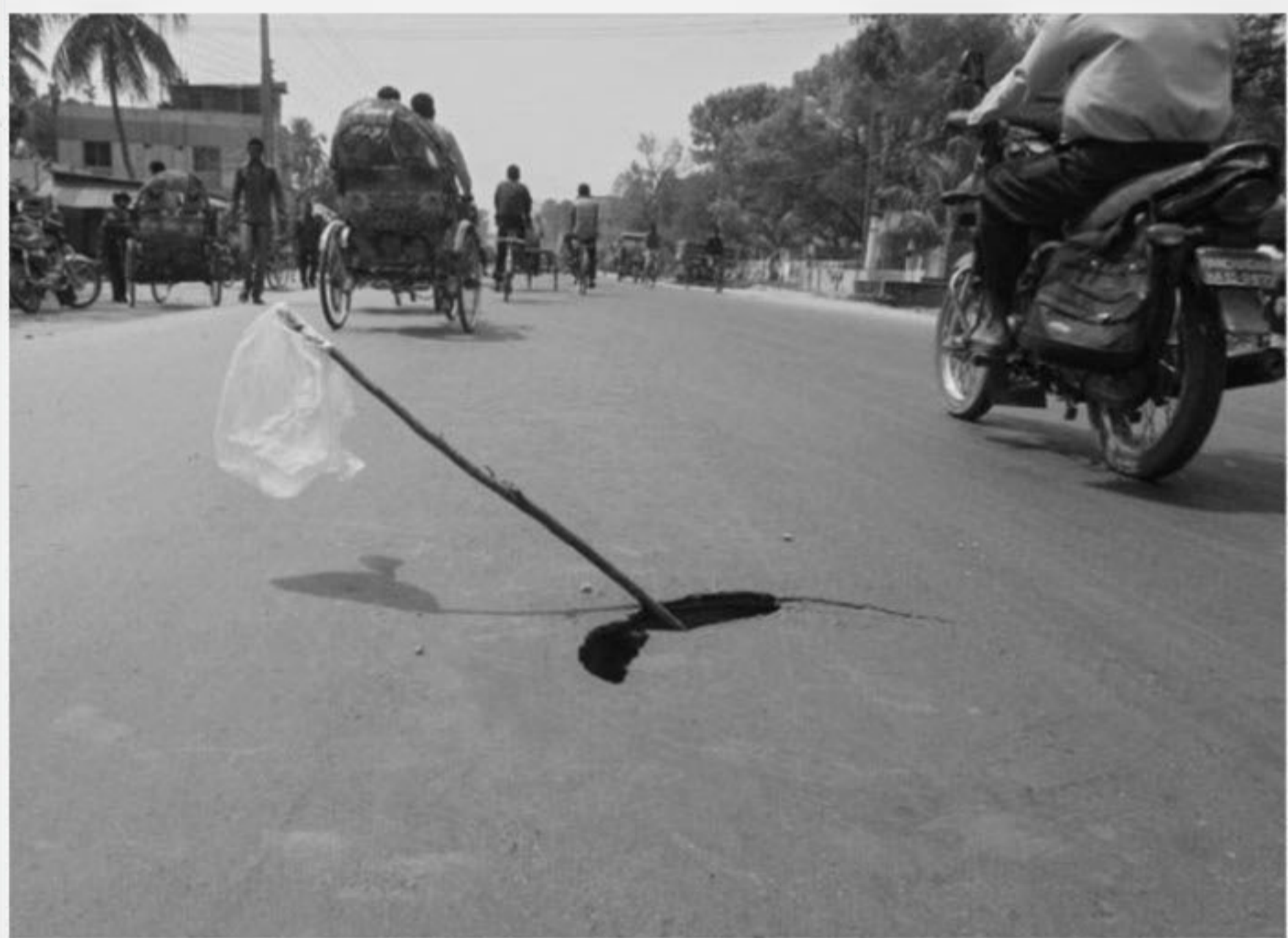
A crack has developed, even before completion of the renovation and extension work on Panchagarh-Banglabandha road, in front of Panchagarh Sadar Hospital, raising question about the quality of the work under Roads and Highways Department.
