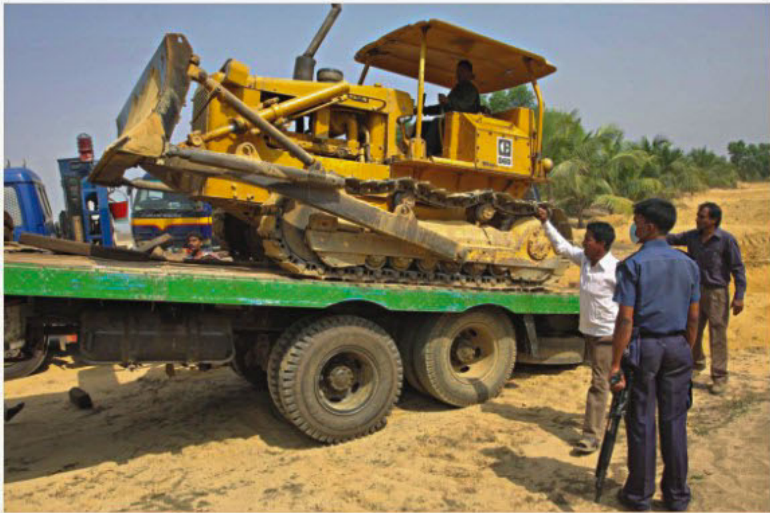
One of the bulldozers seized yesterday at KEPZ in Chittagong. The DoE made the seizure, noting that the construction vehicles were being used in hill-cutting.
