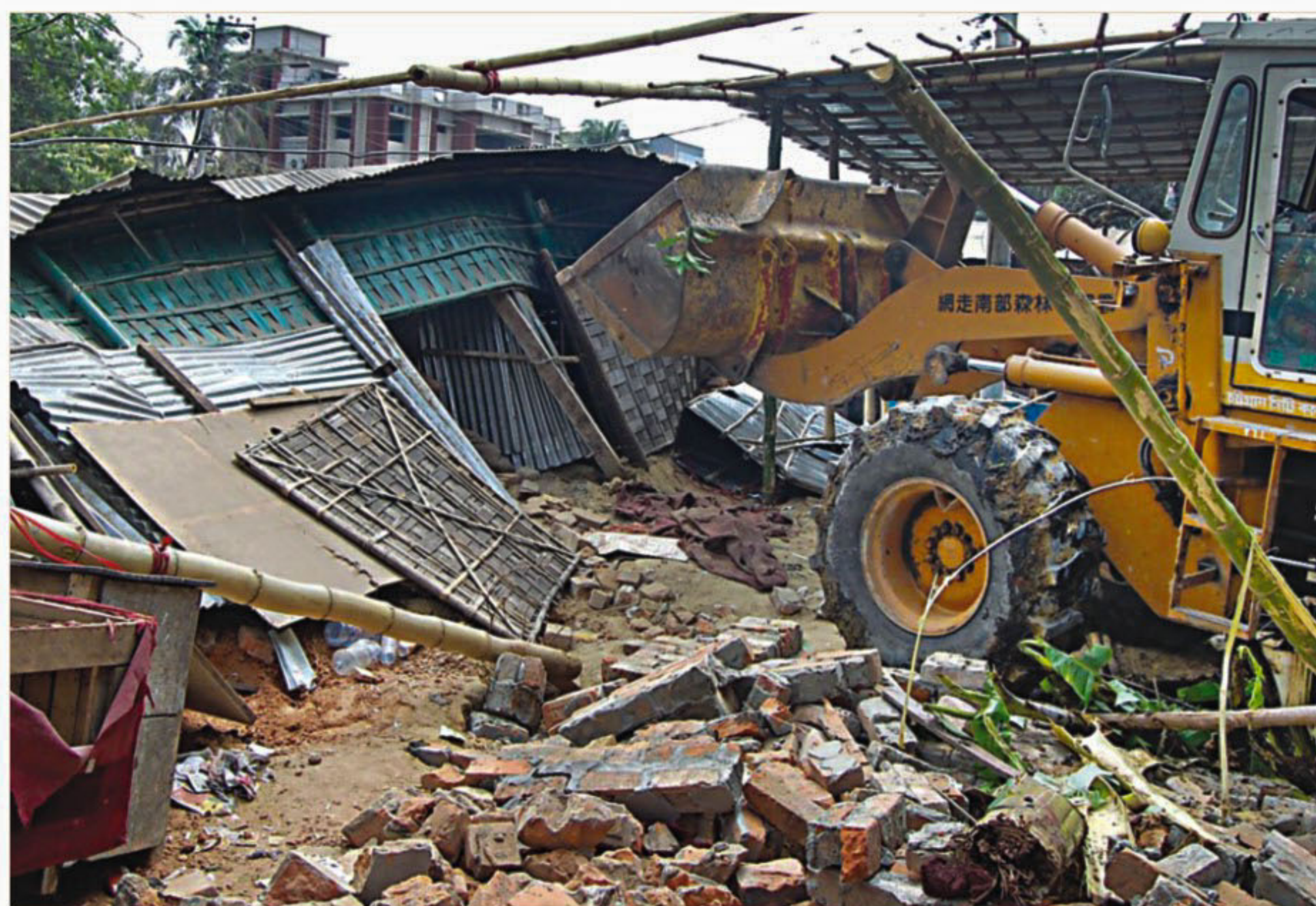
Chittagong City Corporation (CCC) demolishes illegal structures in the port city yesterday.
