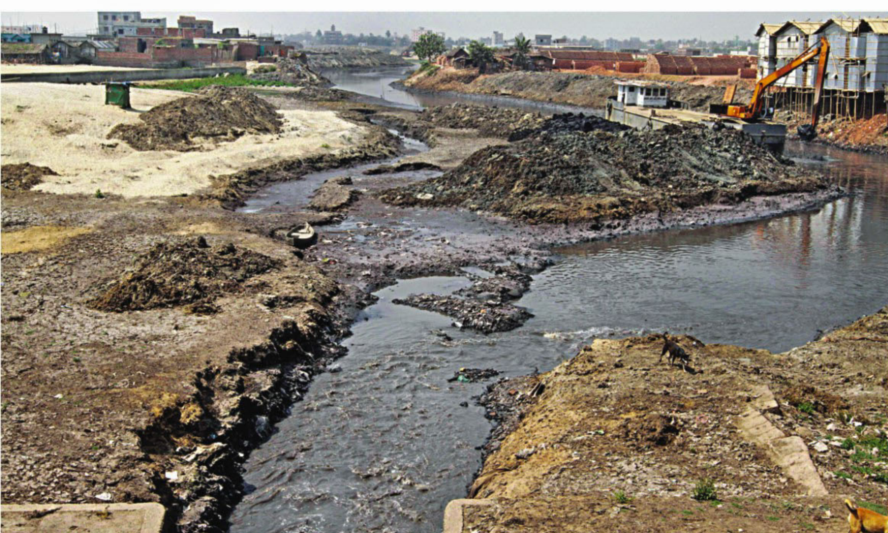
A BIWTA excavator removes soil from a canal in the city's Rayerbazar yesterday to make the water body free-flowing. But the agency dumps the dug-out earth right on the bank, making it possible for the canal to get filled up again. The soil can easily be washed back into the canal.
