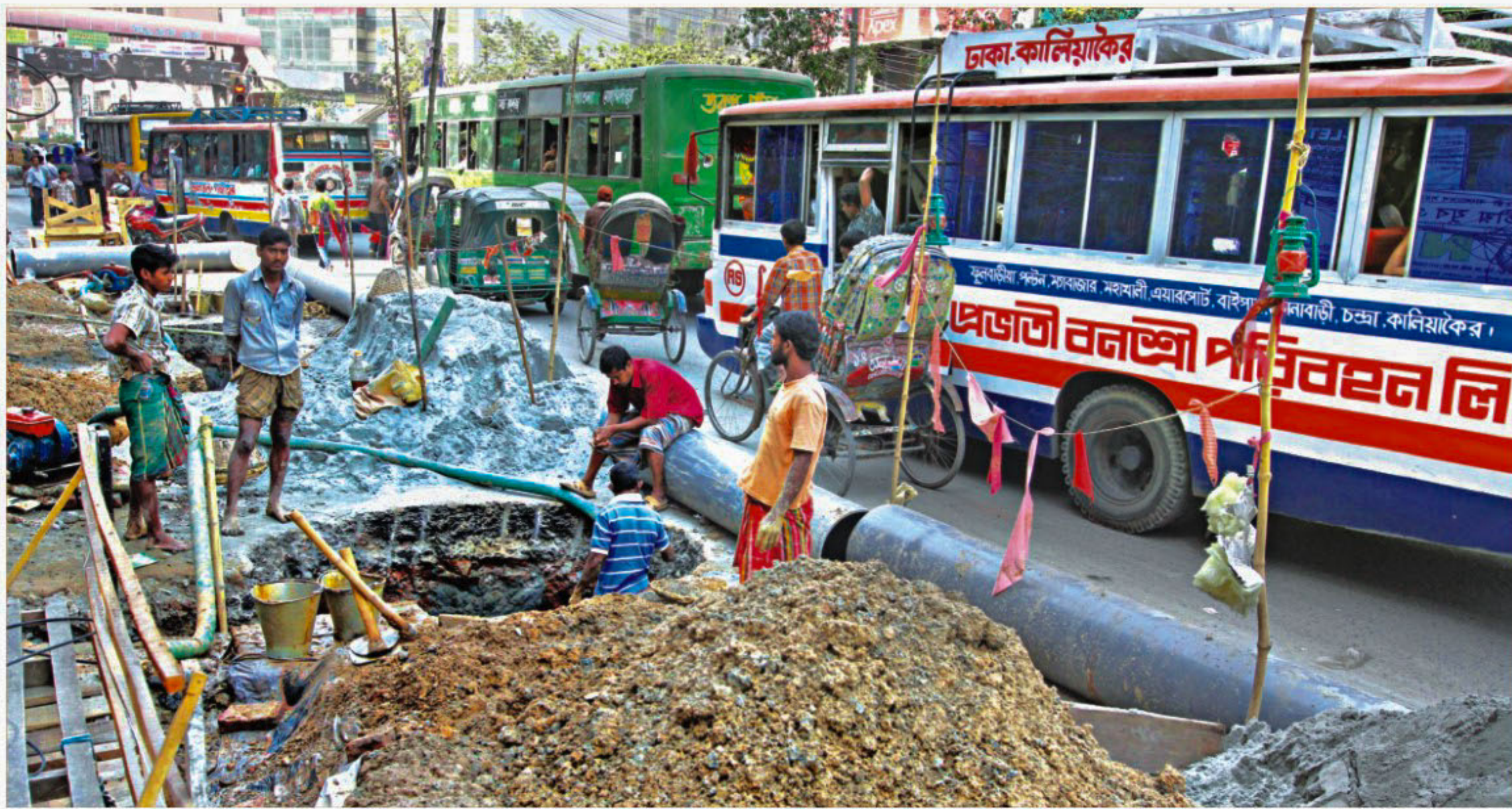
Heaps of soil and big pot holes, in the name of water pipe construction work by Wasa, cover a big portion of New Circular Road near Mouchak Market in the city, creating long tailbacks and sufferings to commuters and pedestrians in the area. The photo was taken yesterday.
