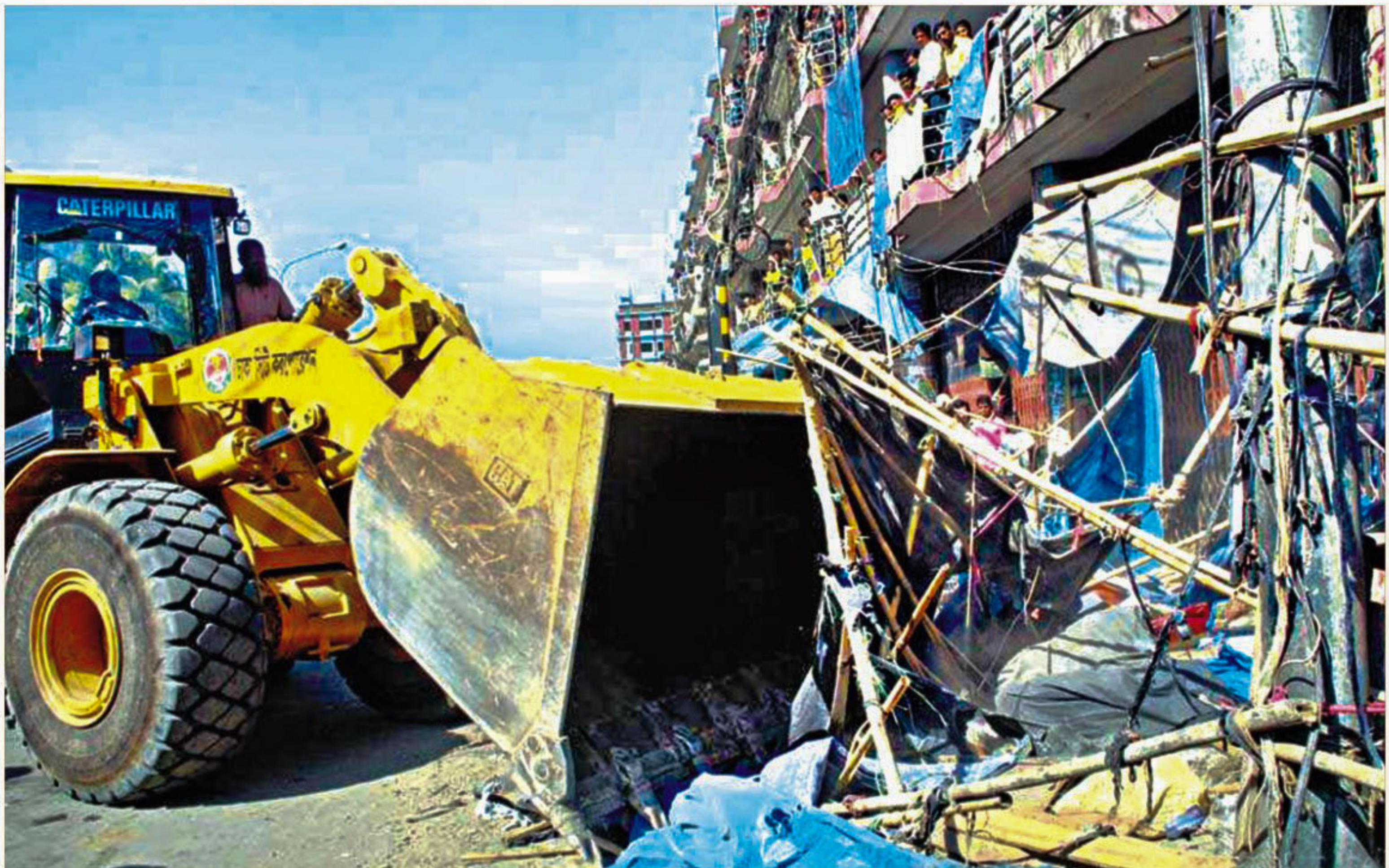
A Dhaka City Corporation bulldozer evicts shops illegally occupying a road in the city's Gulistan yesterday. The High Court issued a directive on Sunday to free the roads and footpaths from Zero Point to Sadarghat in 48 hours to facilitate the movement of people and vehicles.
