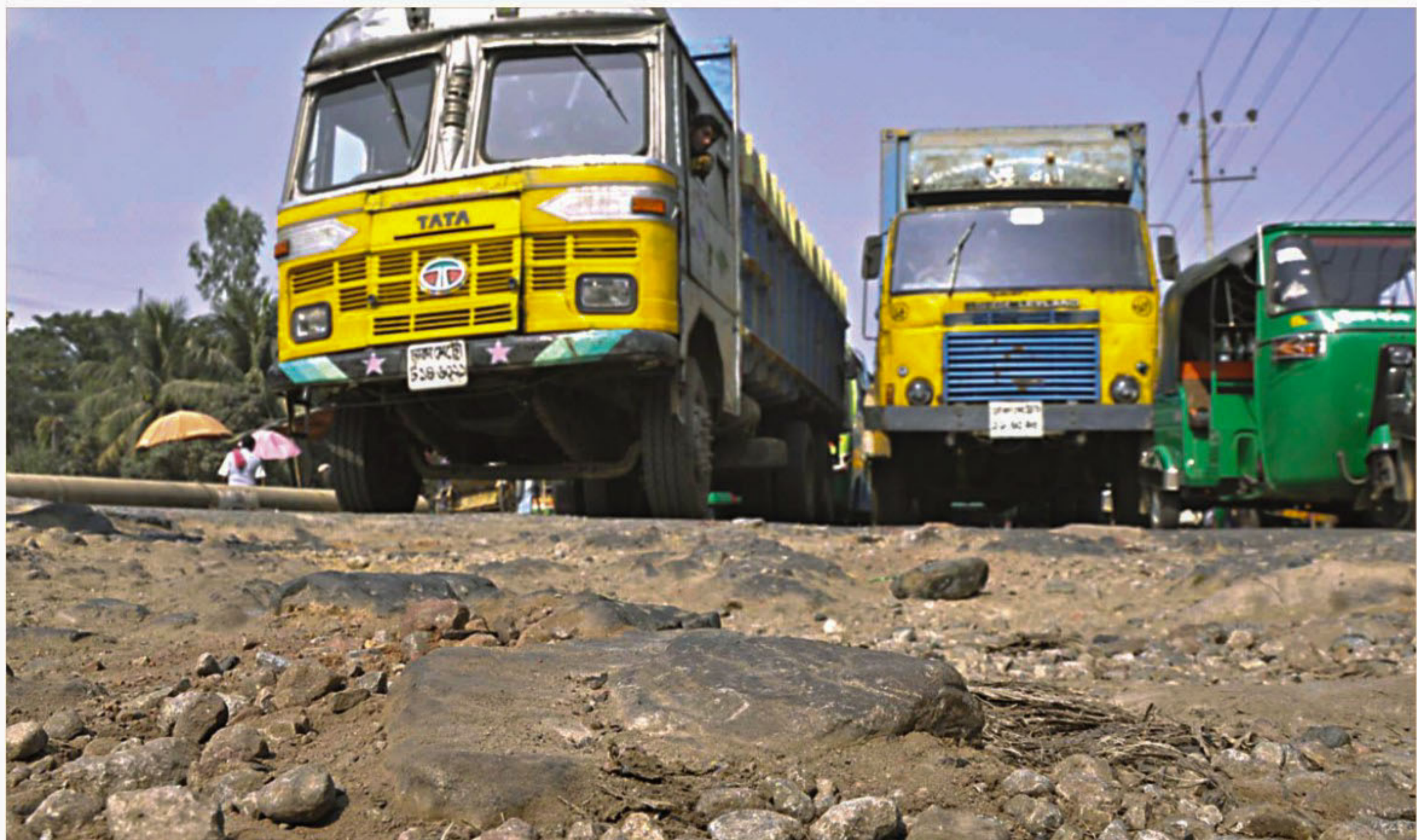
There was a huge outcry from media and transport owners on the battered condition of highways and roads across the country ahead of the last Eid-ul-Azha. But the picture shot yesterday shows this part of Dhaka-Chittagong highway still in very bad shape and almost impassable for vehicles.
