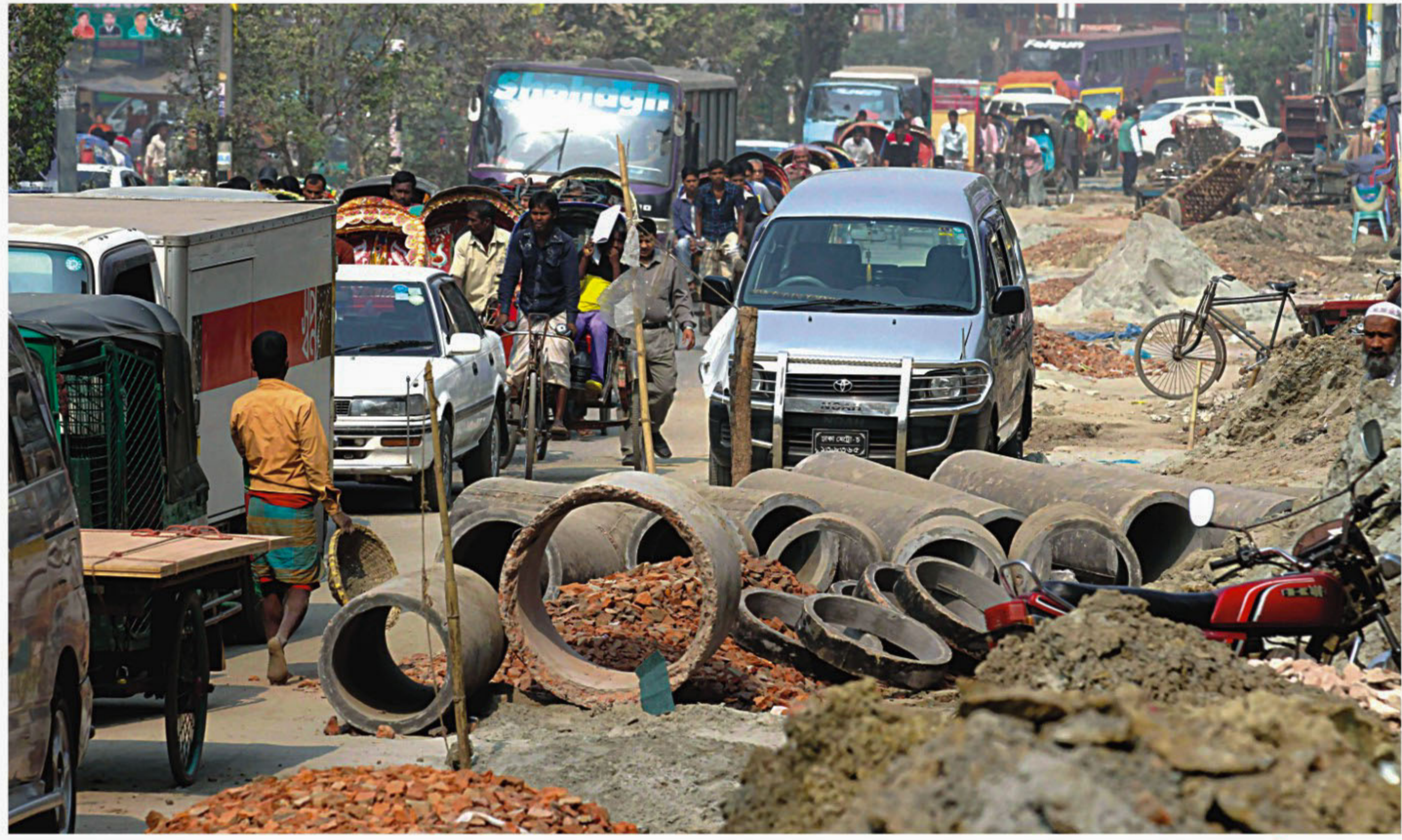
Dhaka Wasa, busy installing sewage lines between Mouchak and Malibagh Level Crossing, has left the pipes and other construction materials on the road. The result: day-long traffic jams on the busy street.
