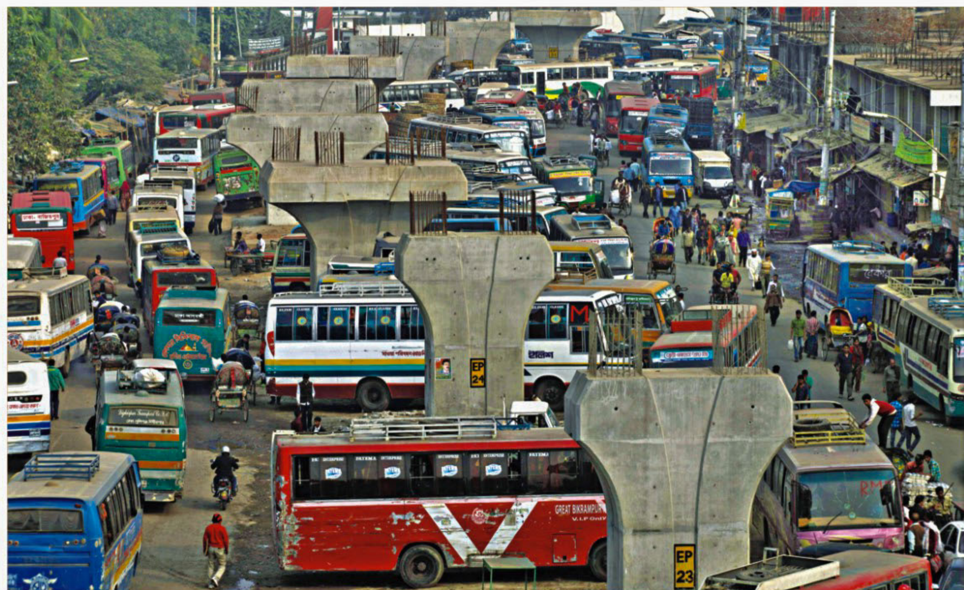
Bus drivers take advantage of the under-construction state of Gulistan-Jatrabari flyover to keep their vehicles parked between the supporting pillars in Kaptan Bazar area of the city, obstructing a free flow of traffic. PHOTO: RASHED SHUMON
