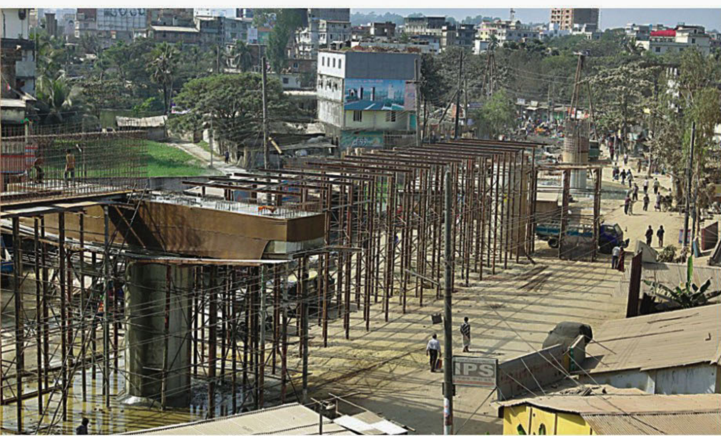
The construction of Bahaddarhat flyover in Chittagong has closed the road to traffic while people are left to wait patiently for the slow-paced work to end. The photo was taken on Tuesday.
