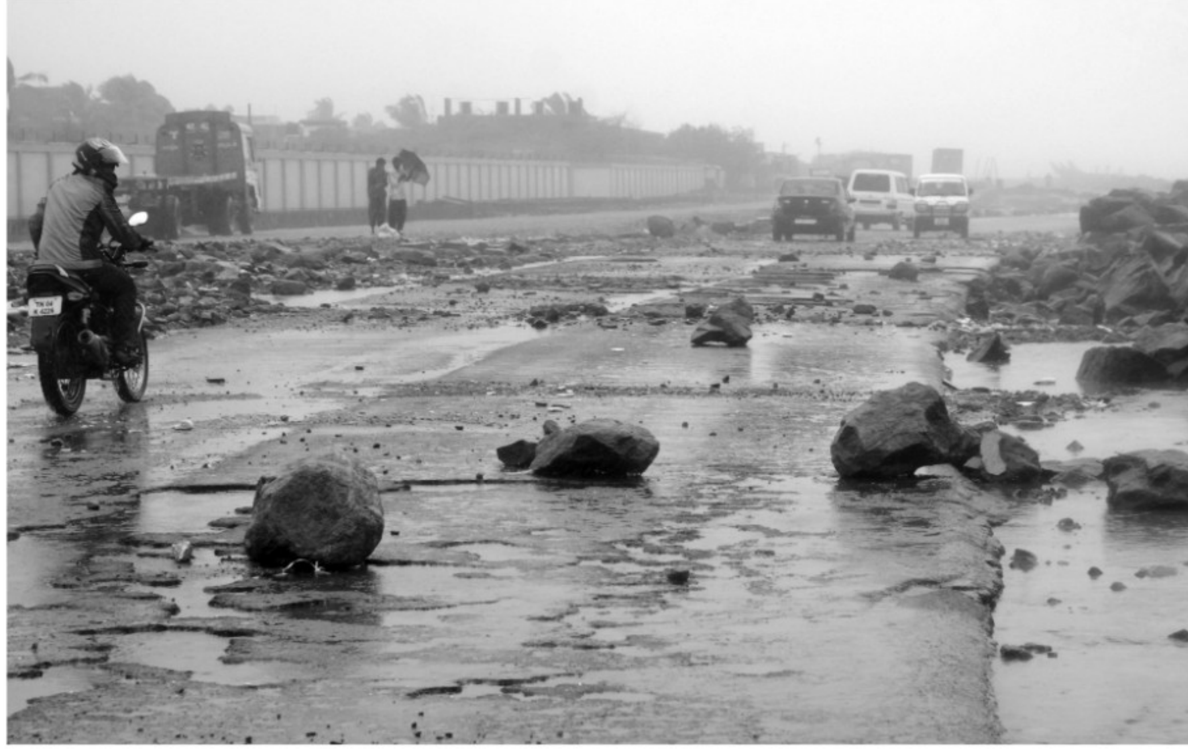
A man rides a motorbike on a damaged highway along the Bay of Bengal Sea on the outskirts of Chennai after Cyclone Thane hit the southern Indian state of Tamil Nadu yesterday.
