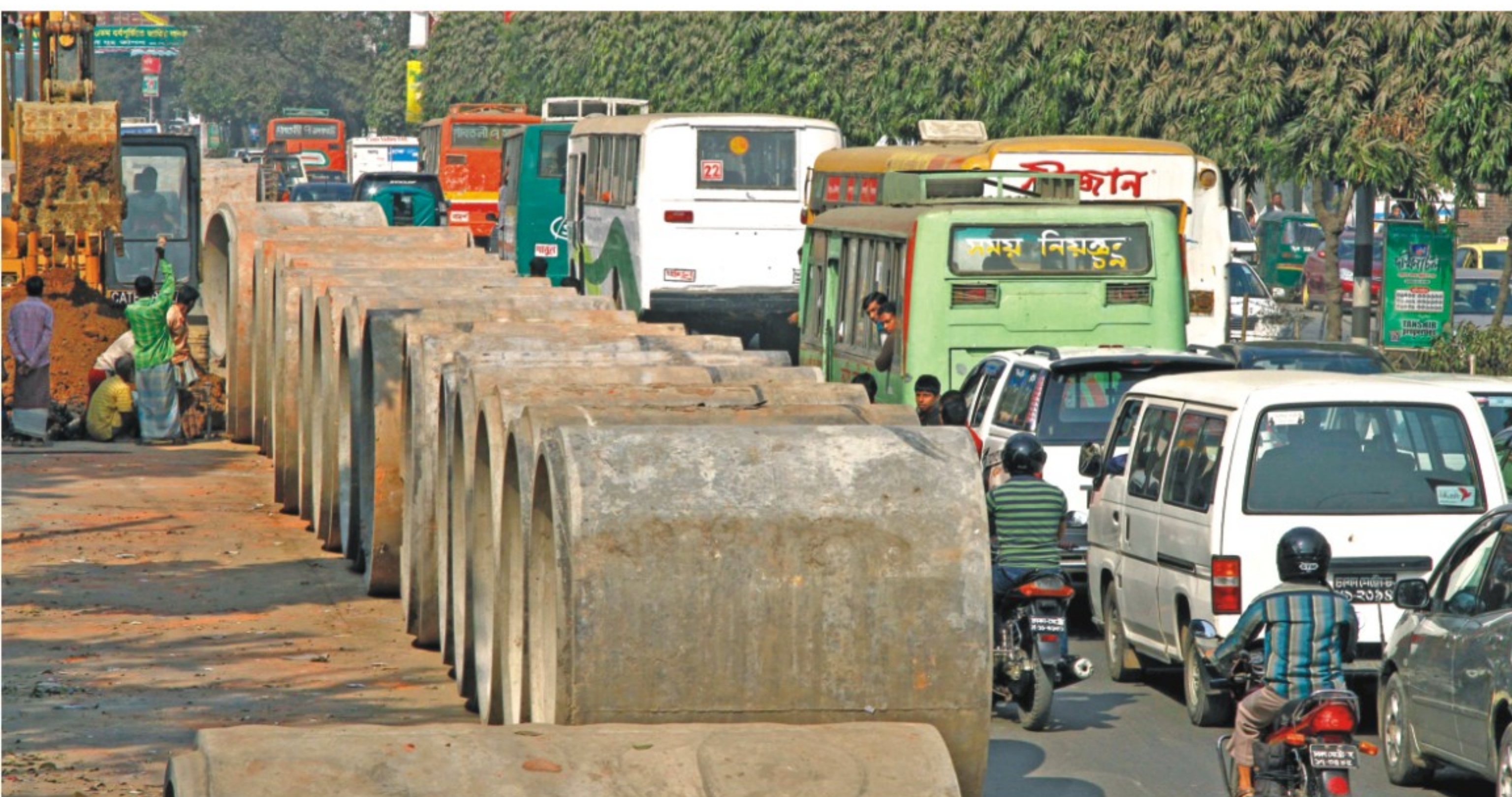
Segments of sewage pipes, waiting to be installed, are narrowing down the busy Mirpur Road in the capital's Dhanmondi area and obstructing traffic. The photo was taken on Thursday.
