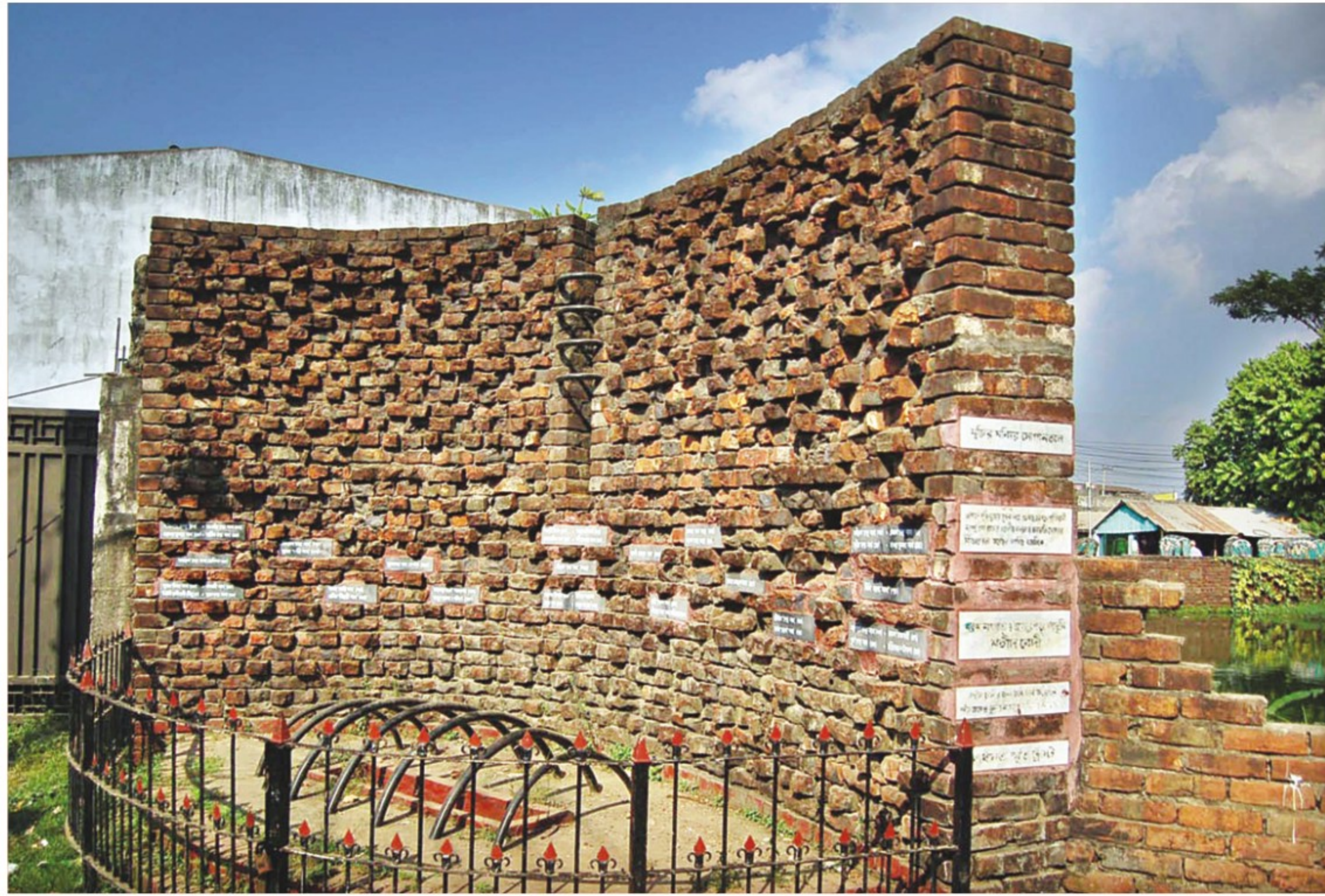
A dilapidated memorial at Modhyam Nath Para of Halishahar in the port city.
