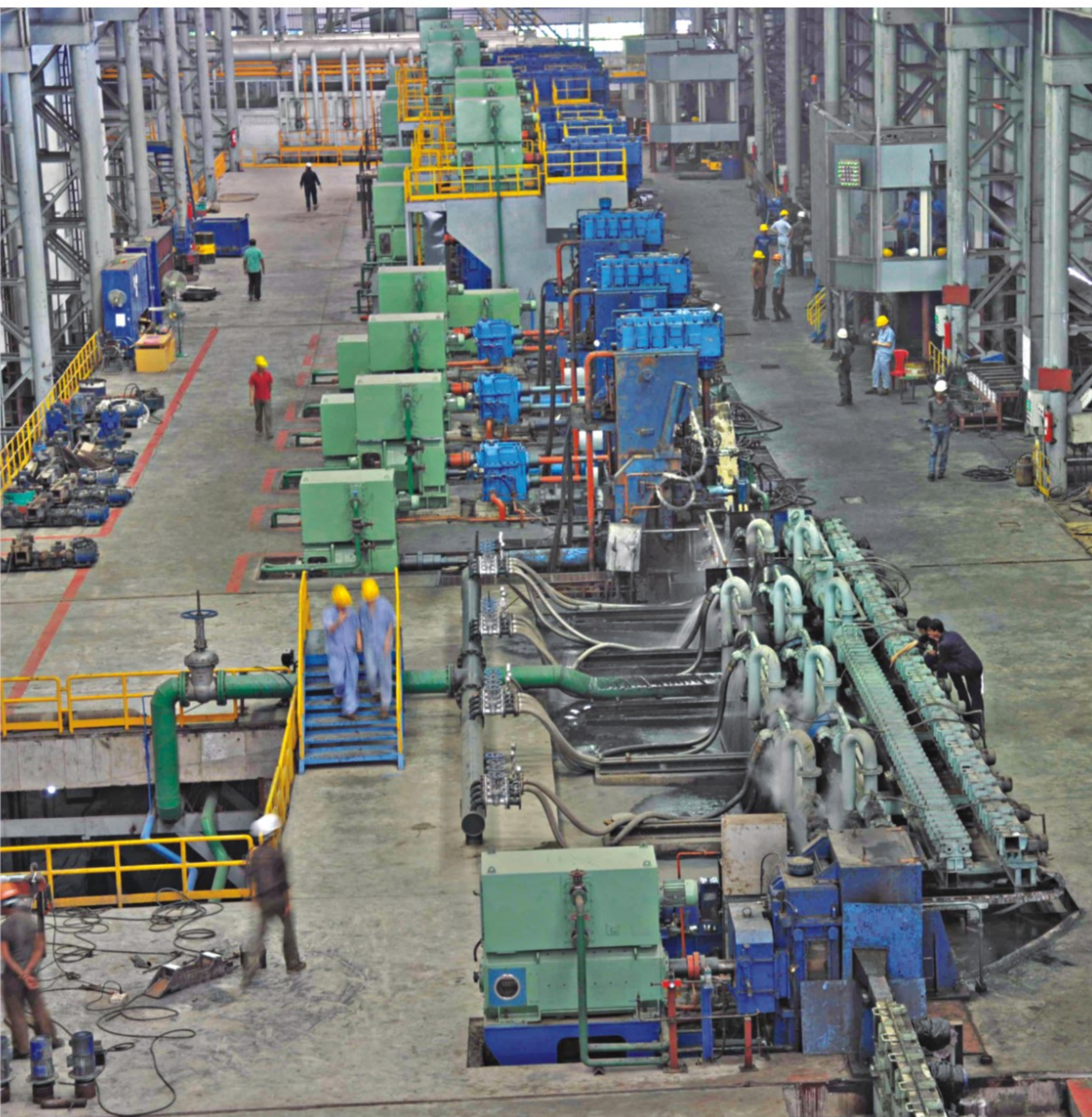
TMT Processing unit
