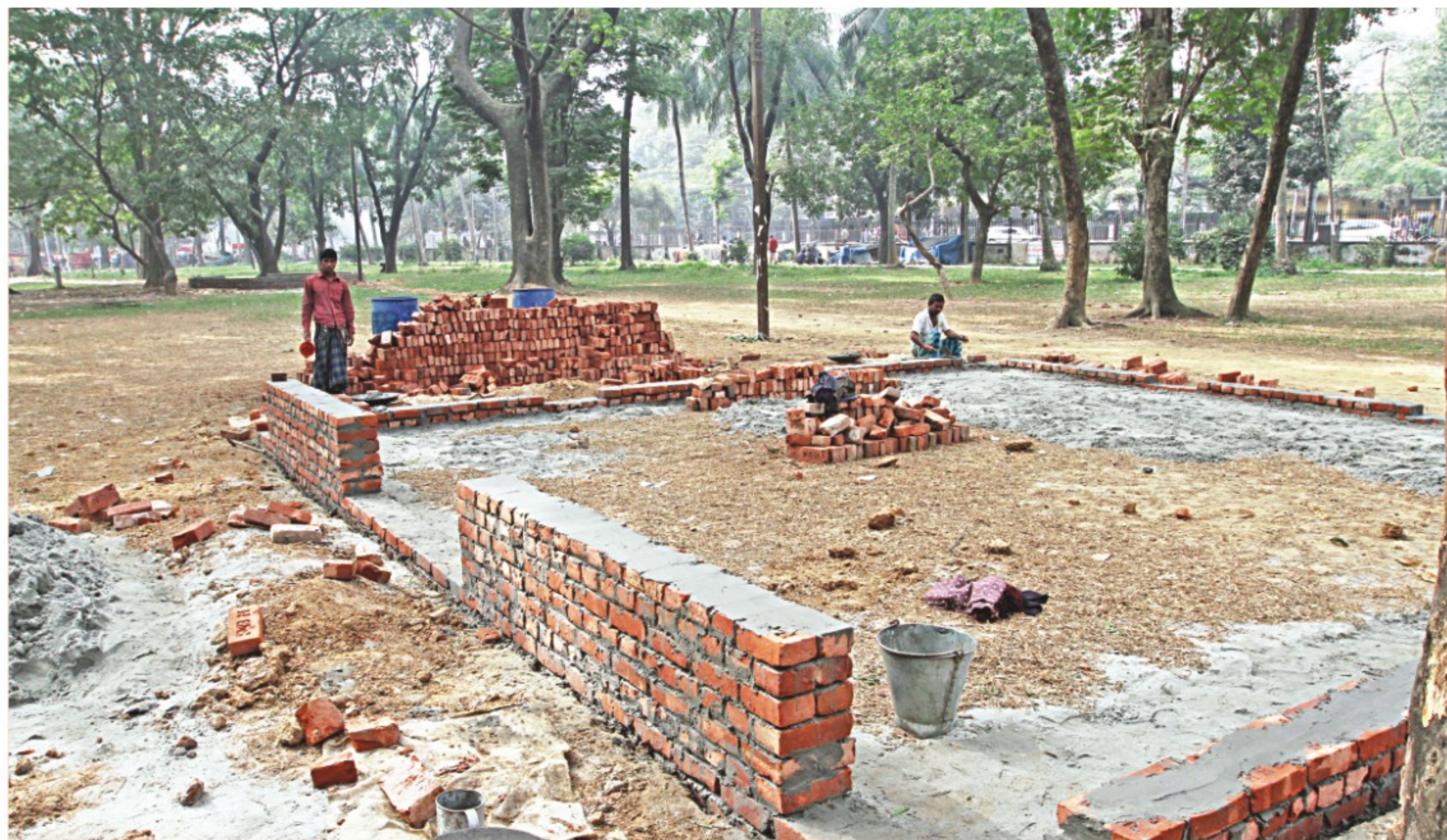
Construction of a seating arrangement for visitors going on at Suhrawardy Udyan in the city in the absence of a comprehensive development plan for the grounds. The photo was taken yesterday.
